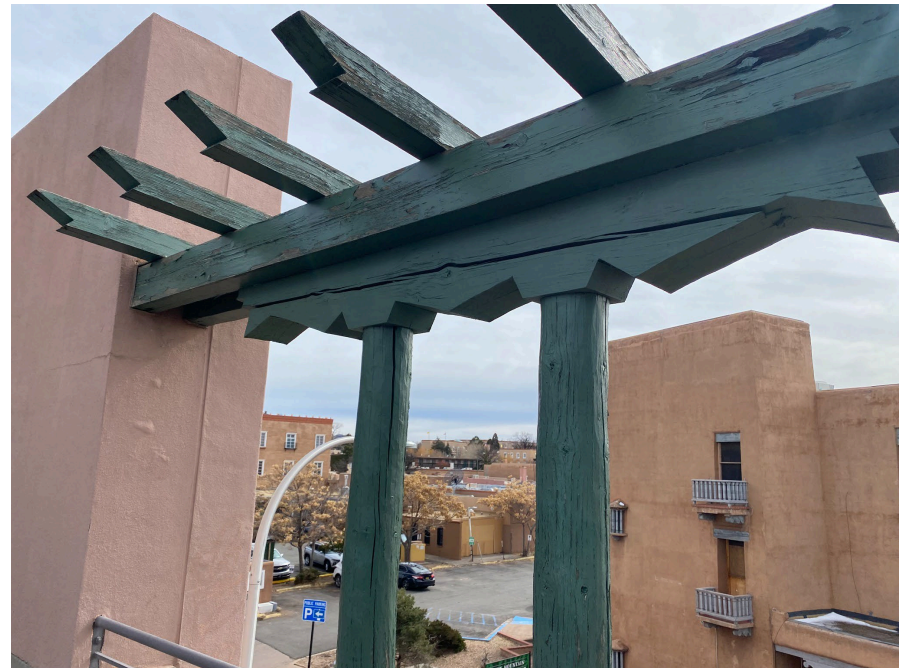
Existing beam conditions with visible weathering and deterioration.
