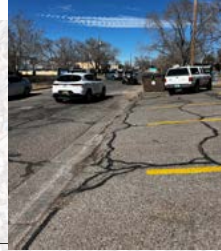
Street missing sidewalks
