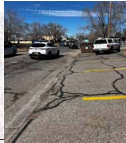
Street missing sidewalks
