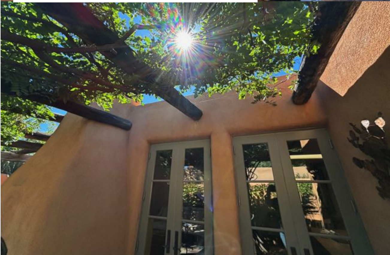
ROTTEN PERGOLA STRUCTURE TO BE REPLACED - NON-HISTORIC MATERIAL TO THE EXISTING HOUSE BUT WAS ALL RECLAIMED BARN WOOD THAT HAS STARTED TO CRACK AND BEND.
