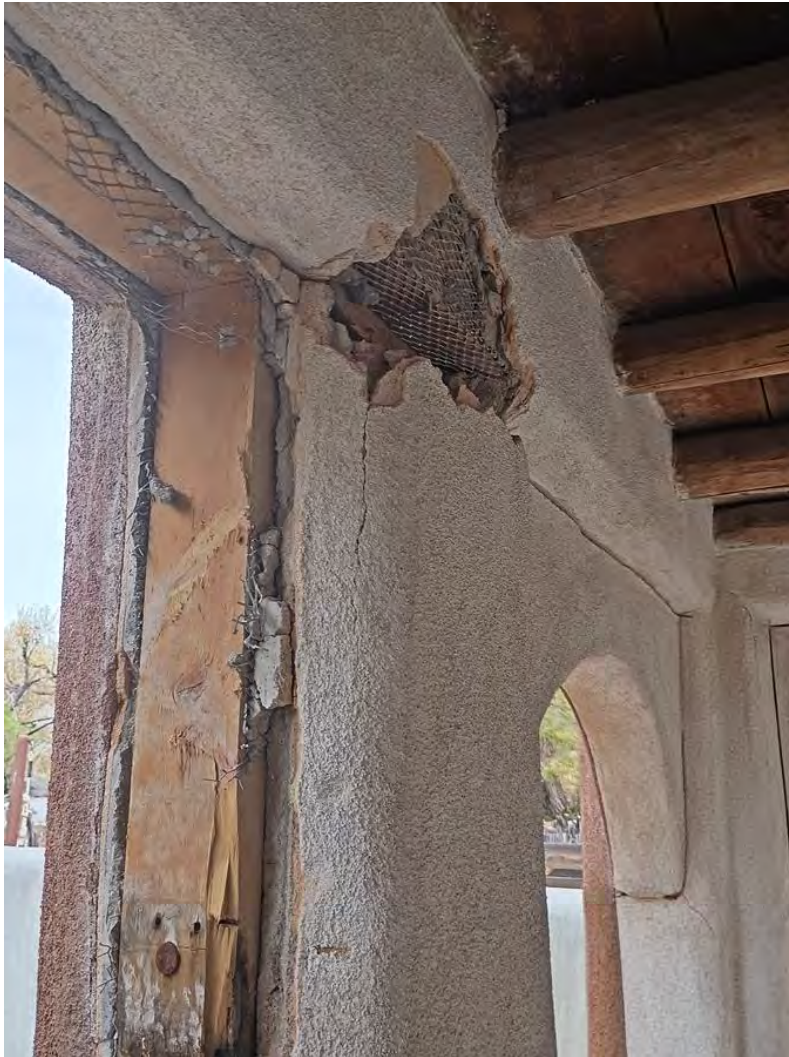
Photo 5: North façade entry portal, damage to plaster. Camera facing up.
