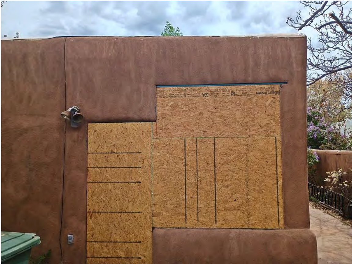
Photo 9: North façade, former entry and window of solarium filled in with OSB sheathing. Camera facing south.
