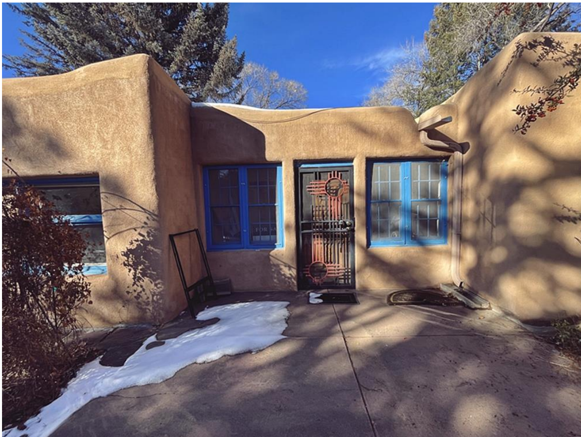
Photo 3: East Elevation. Entry. Enclosed entry hall was constructed in 1954. Camera facing west.
