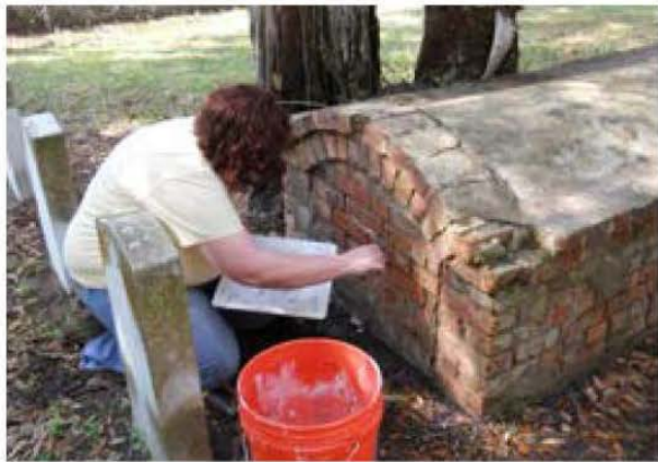
Figure 19. Masonry markers like this box tomb may require the repointing of mortar joints. It is important to use a mortar that is softer than the historic brick. In this case a conservator uses a lime putty-based mortar to repoint. Photo: Jason Church.
