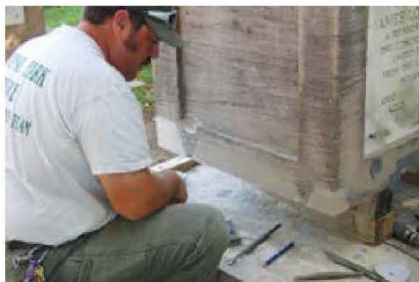
Figure 16. A professional mason works to insert a new piece of stone. Often referred to as a "dutchman", this repair technique requires replacing the deteriorated stone section with a new finished piece of the same size and material. Photo: Jason Church.
