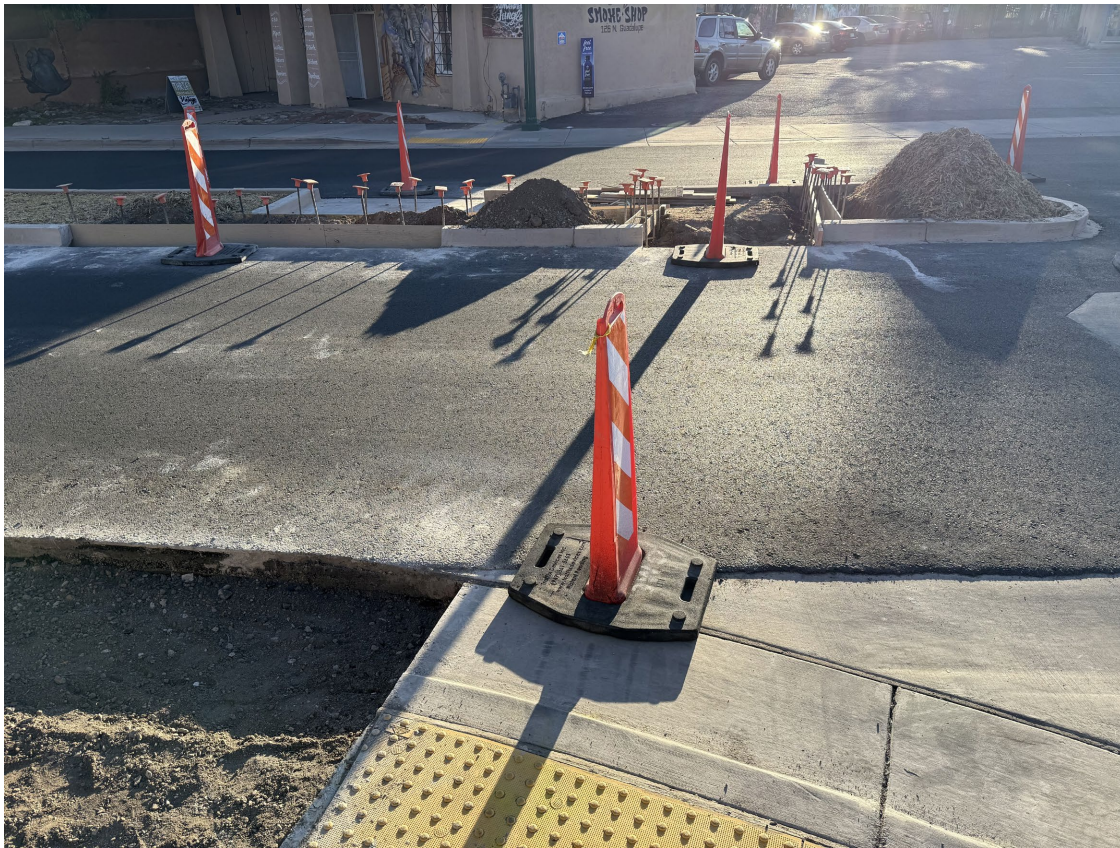
Curb removed to accommodate faster traffic, looking south at Guadalupe St and Agua Fria
