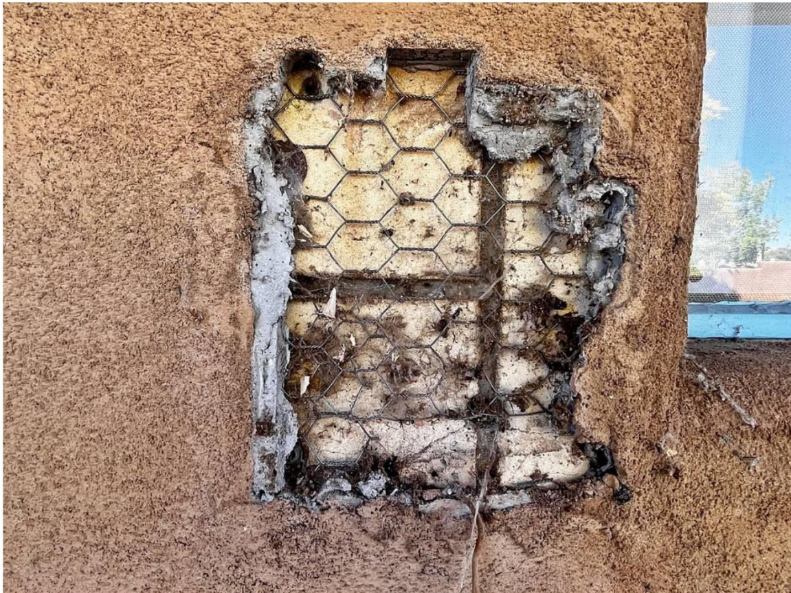
Photo 11: East elevation. Whit veneer cladding behind electrical box. Camera facing west.
