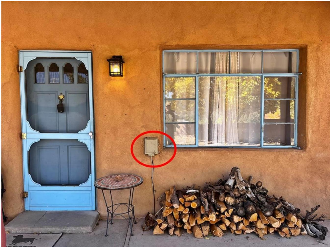
Photo 10: East elevation. Entry to living room. Electrical box circled. Camera facing west.
