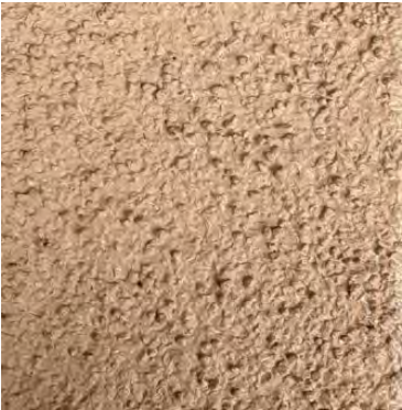
Existing Stucco Locations: La Habra Cementitious Stucco custom color match to Sherwin Williams SW9097 Soft Fawn
