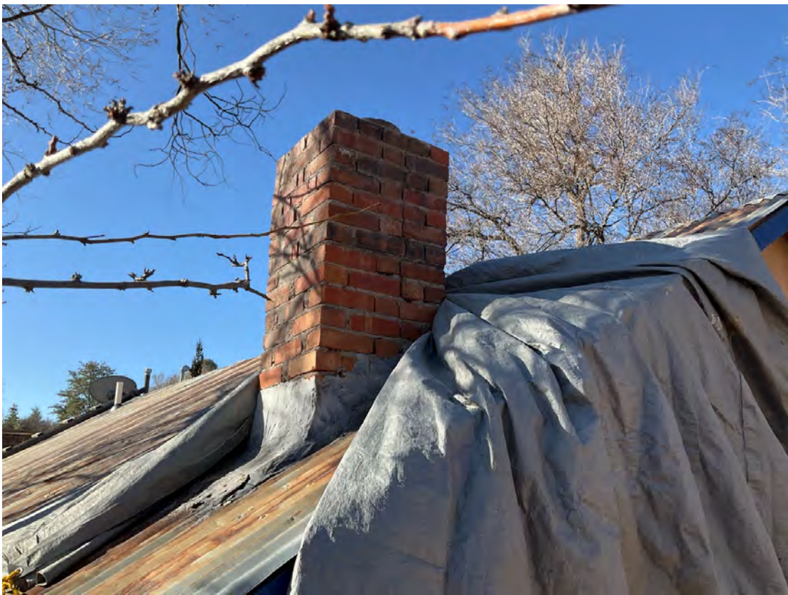
Chimney termination does not have cap. Cap is needed to keep out moisture and animals.
