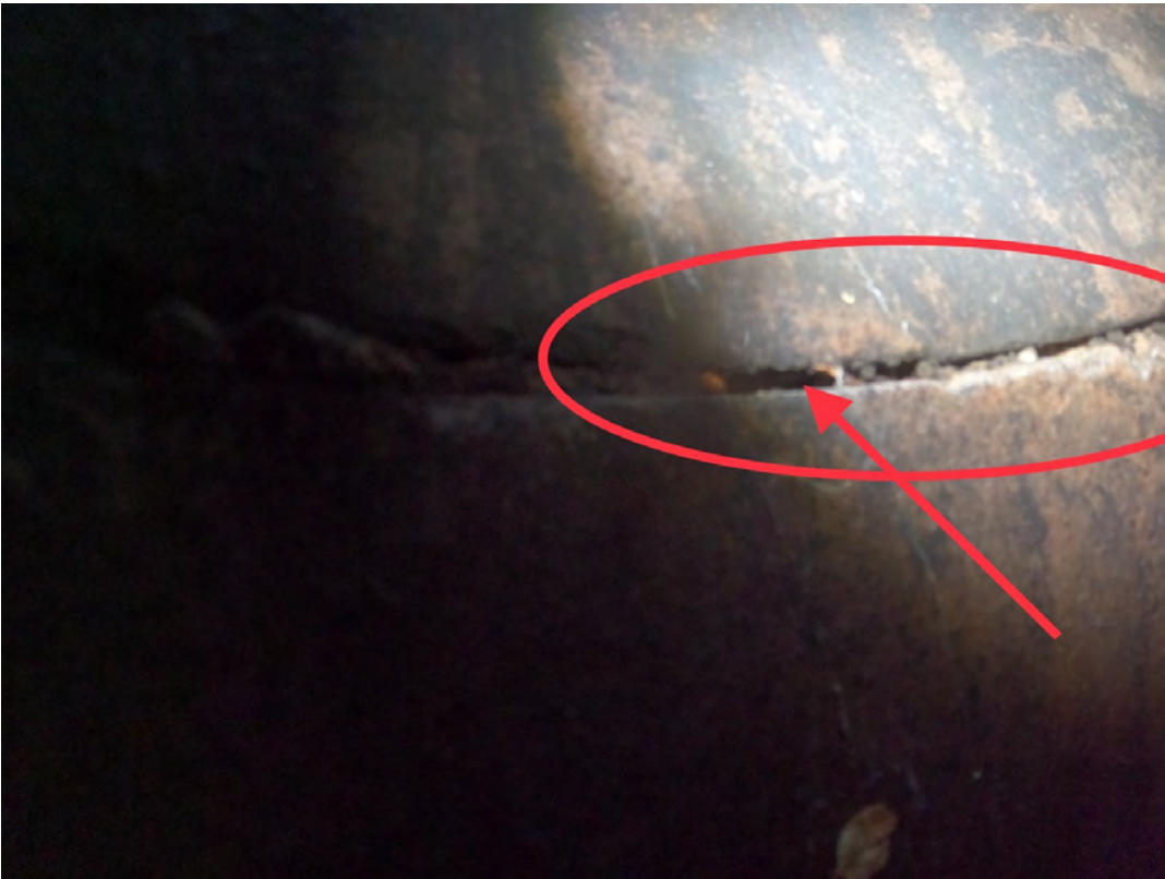
Potential gap between joint sections.
