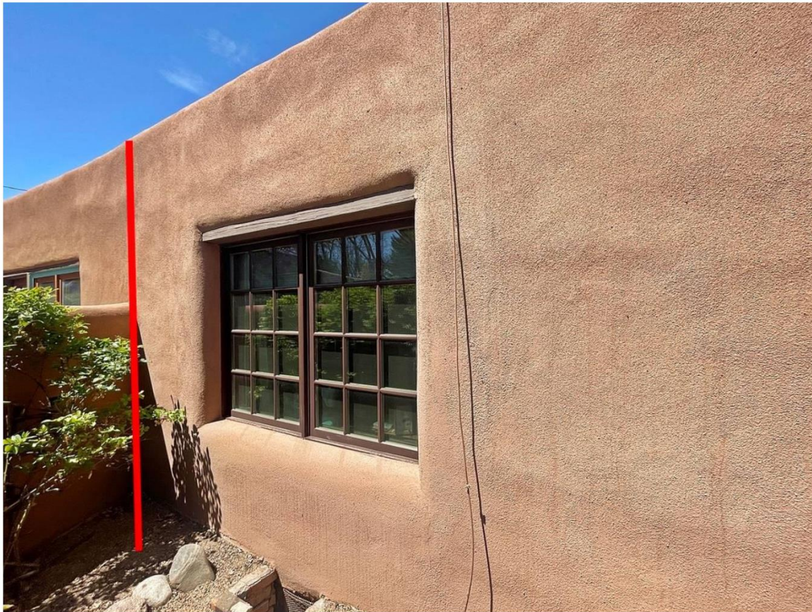
Photo 14: South elevation. Window at bedroom. Camera facing northwest. Red line indicates end of subject of condominium and the beginning of Unit 3. April 20, 2024.
