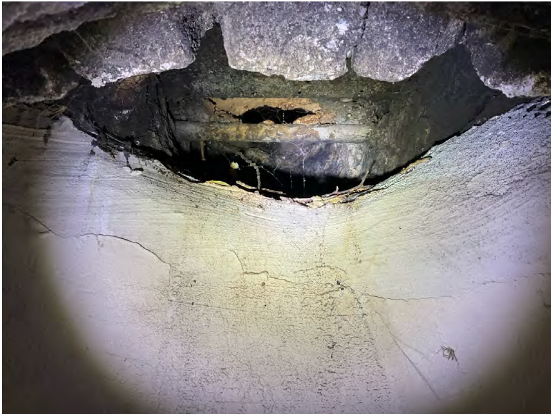
View looking into smoke chamber no damper detected.
