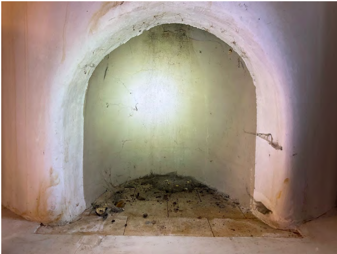
Firebox is plastered with non refractory material and should be rebuilt with refractory brick and mortar.
