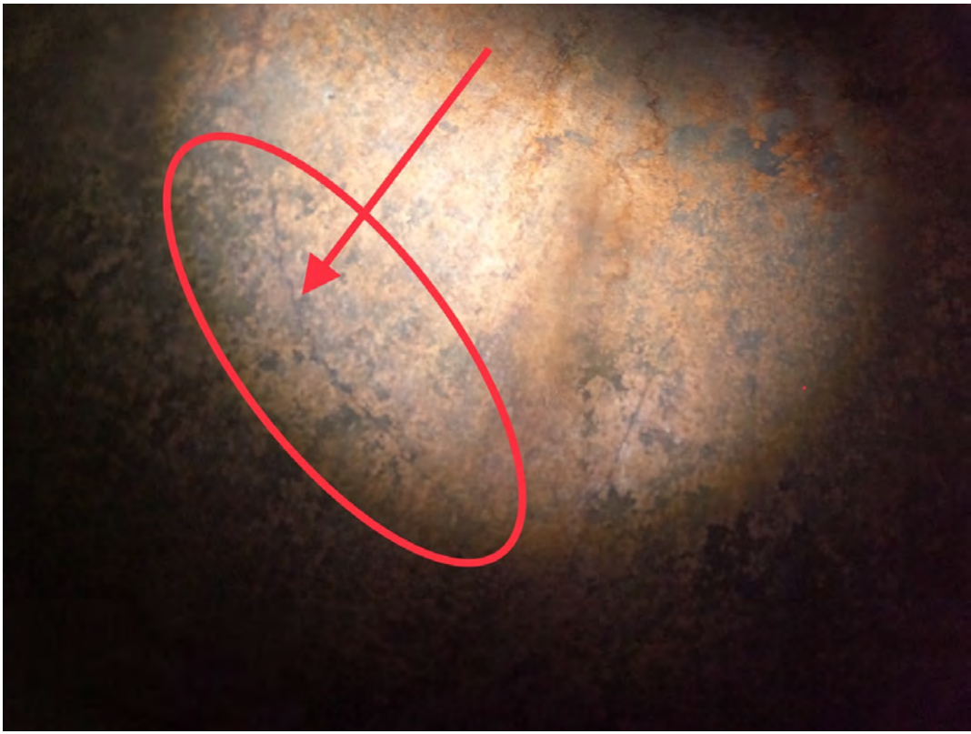
Vertical crack detected in chimney passage.
