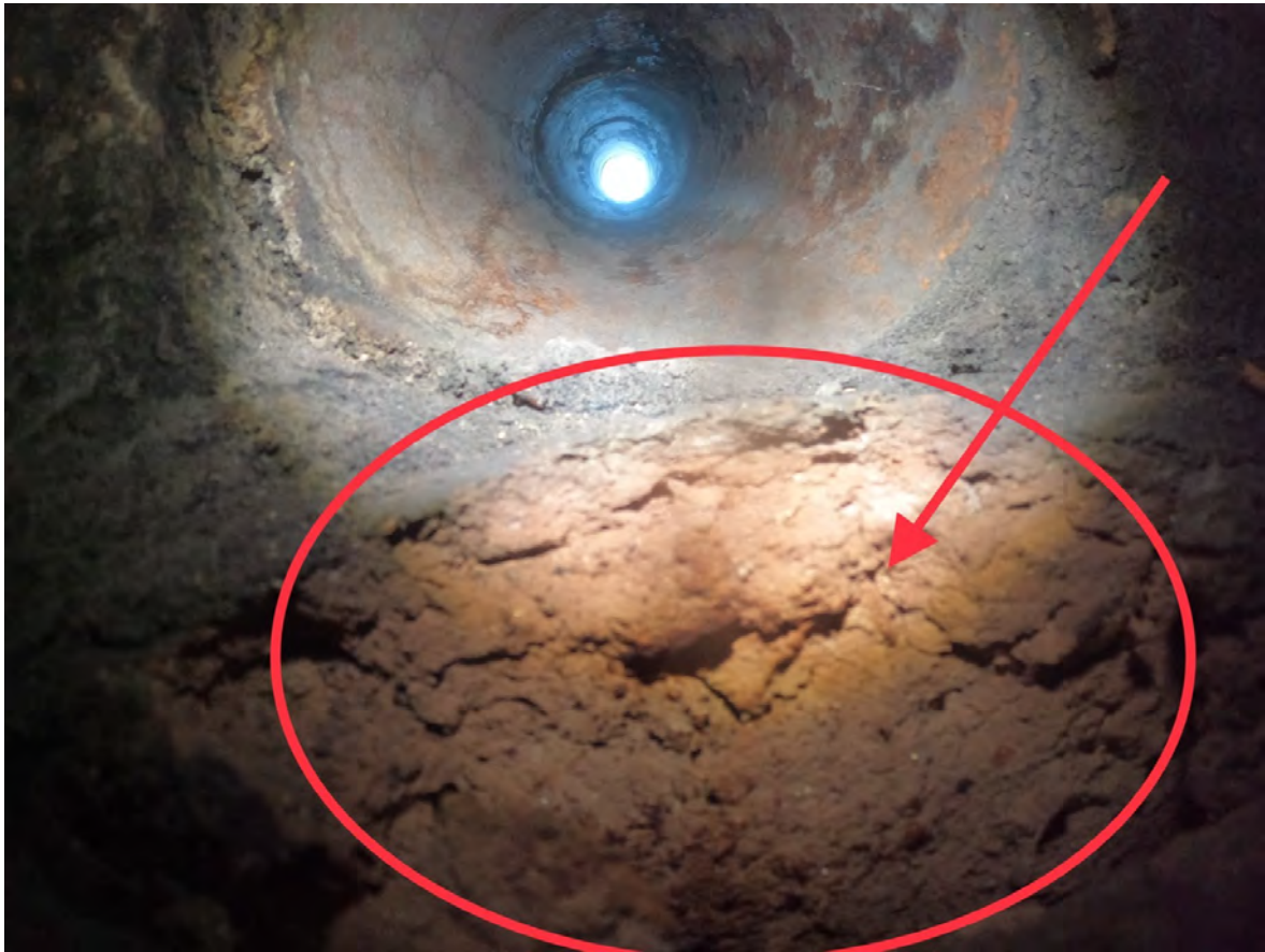
Smoke chamber is bare adobe. Smoke chamber should be parged smooth with refractory cement.
