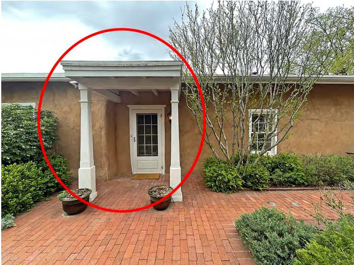
Photo 10: South elevation, entry. Circled porch and door altered in the 1990s. Camera facing north. May 4, 2024.
