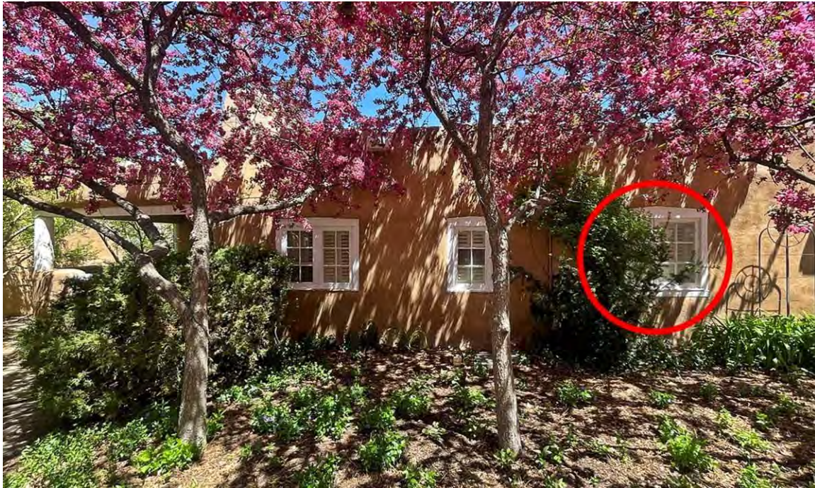
Photo 7: South elevation, west end. Introduced window highlighted. Camera facing north.
