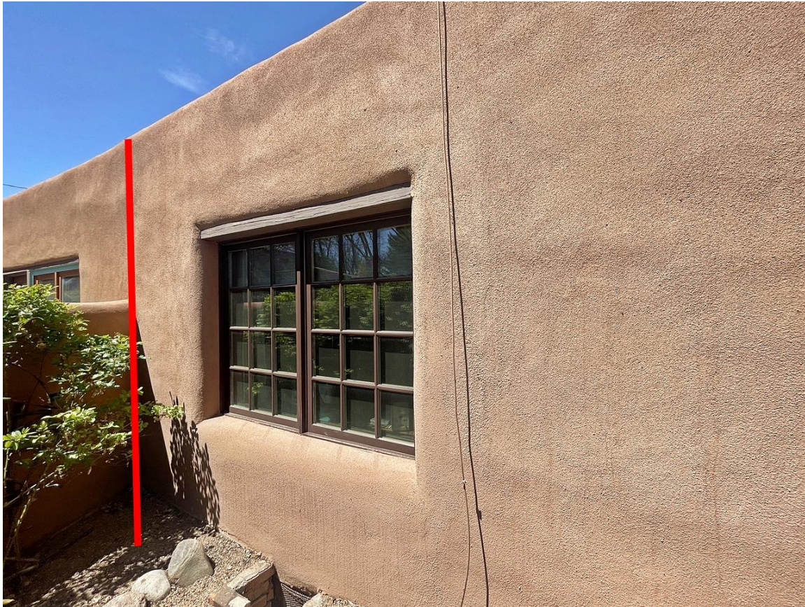
Photo 3: South elevation. Window at bedroom. Camera facing northwest. Red line indicates end of subject of condominium and the beginning of Unit 3. April 20, 2024.
