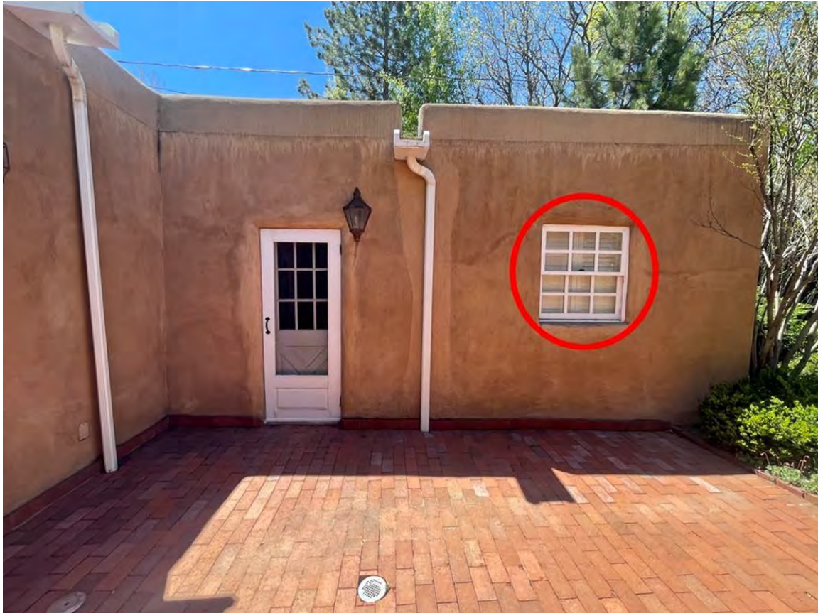
Photo 25: North elevation, 1980s window circled. Camera facing south.
