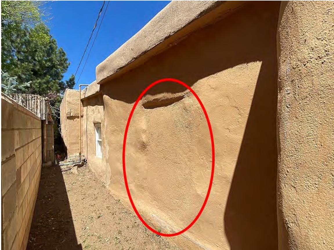
Photo 29: South elevation, middle section. Filled in opening circled. Camera facing northwest.
