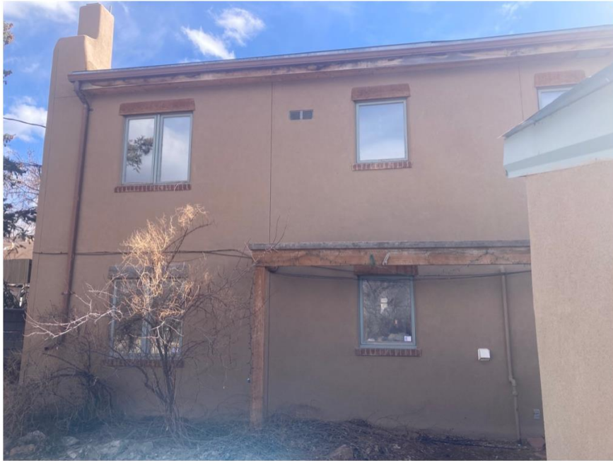
1072 Camino San Acacio, North elevation (left side). View from private yard. This section of the wooden trellis will be repaired/replaced with same.
