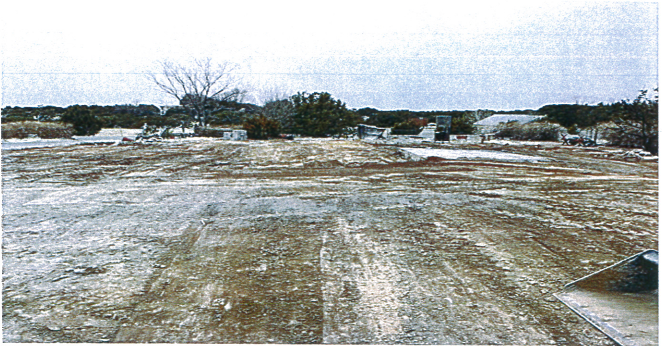
Photo No. 4 Another view of property after the house demolition. Photo taken 3/8/24.
