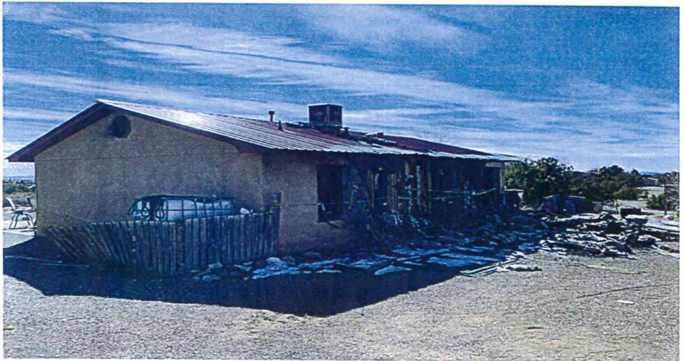
Photo No. 2 Rear view of burnt house. Photo taken 2/20/24.
