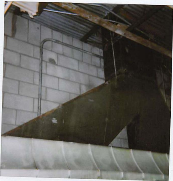
58 E. SAN FRANCISCO 10/26/00 MASONRY wall ASSY WITH OLD MECHANICAL PART. 10/26/00
