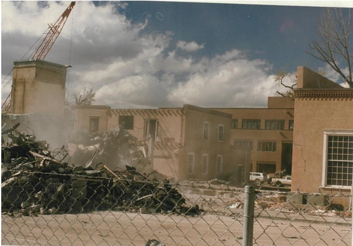
Figure 12: Demolition of center block and 1960s southeast corner addition. Construction photographs, November 11, 1985. Courtesy City of Santa Fe.
