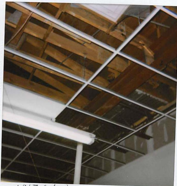
10/26/00 58 E. SAN FRANCISCO 10/26/00 WOOD FRAME MAKE SHIRT TRUSS ASSY CEILING ASSY 1ST FLOOR
