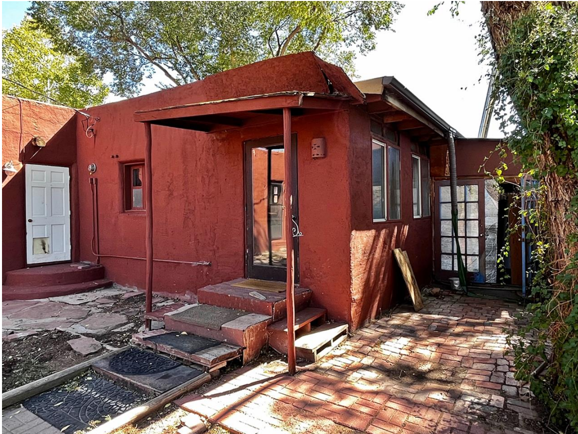
Photo 6: North and west elevations of post-1978 porch enclosure. Entry to shanty at right. Camera facing southeast.
