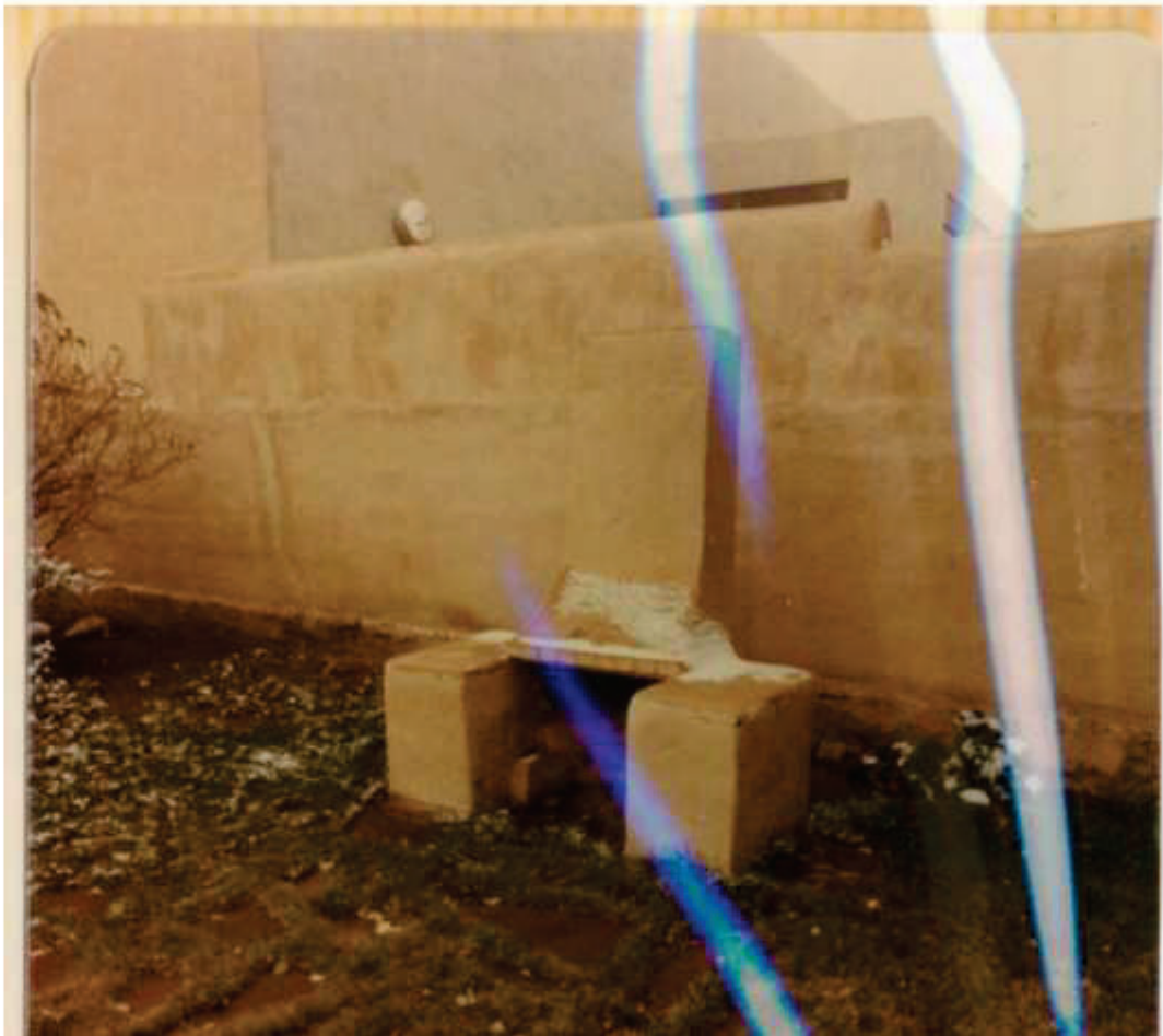
Figure 28: East-West Wall and fireplace, October 28, 1976. 135 Grant Avenue Family Album. Source: Private Collection. Image courtesy of the Georgia O’Keeffe Museum, Santa Fe, New Mexico. Note that the wall appears to be added upon in height.
