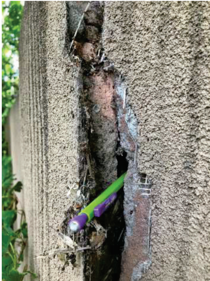
Figure 24: Delamination of “Middle Section,” showing multiple stucco applications. July 2, 2021, John W. Murphey.
