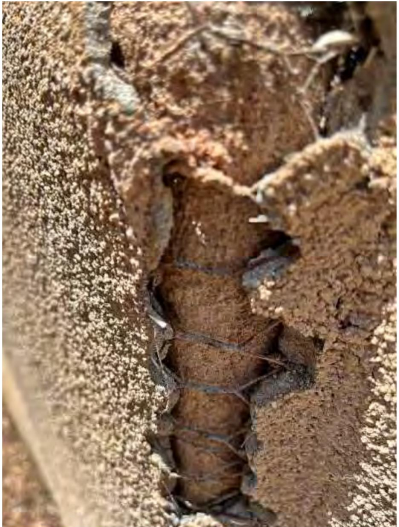
Photo 15: Street Wall, evidence of re-stuccoing. Camera facing southeast.
