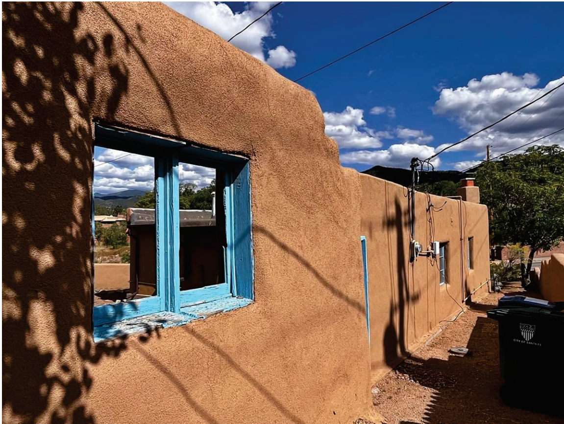
Photo 16: Orphan wall and south elevation of house. Camera facing northeast. October 4, 2023, JWM.
