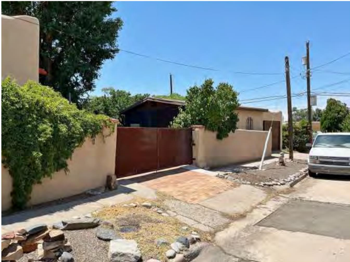
Photo 13: Street Wall, West Buena Vista, likely representing altered section. Camera facing southeast.
