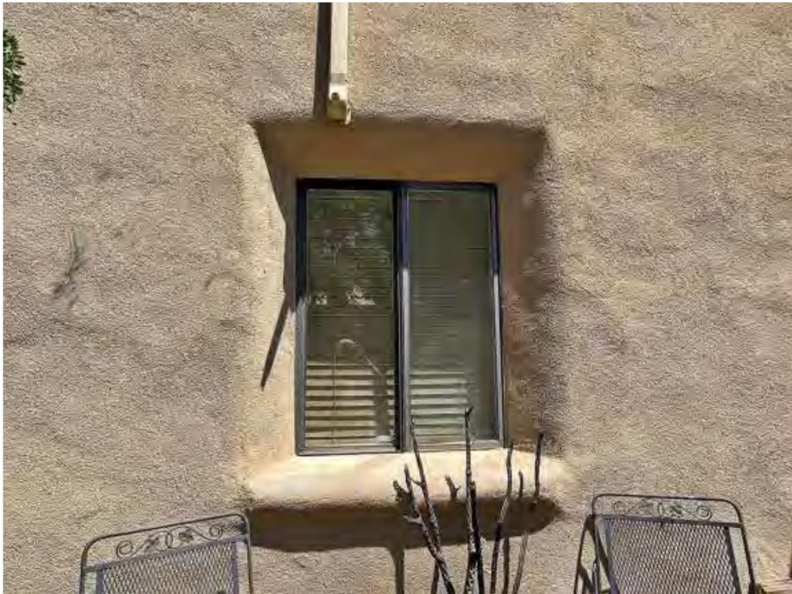
Photo 10: South elevation with typical window with exaggerated reveals and sill. Camera facing north.
