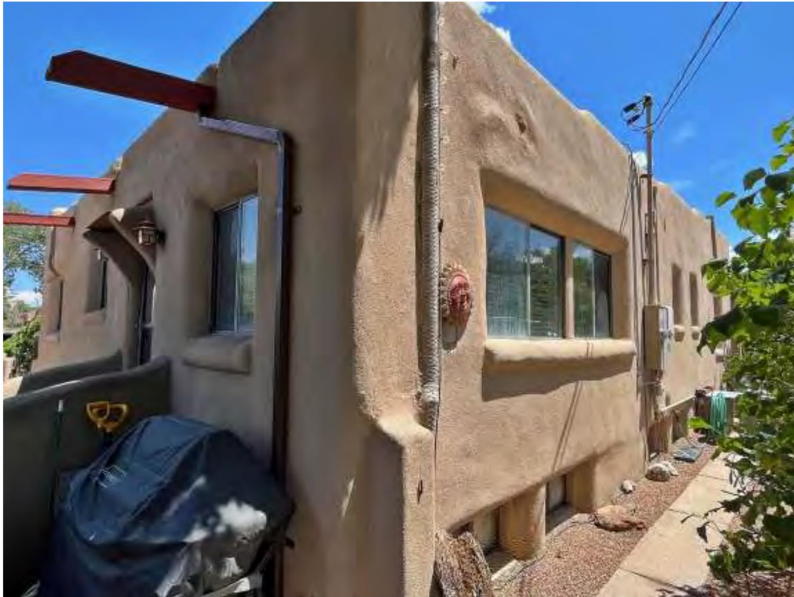
Photo 8: Southwest corner. Camera facing northeast. Note exaggerated window reveals and sills.
