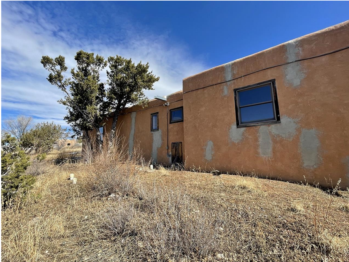
Photo 8: North half and portion of south half of west elevation. Camera facing northeast.
