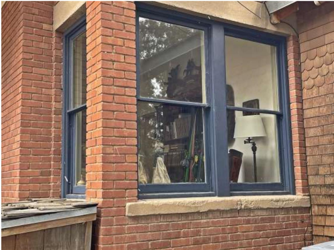
Photo 5: Older 1/1 windows at south and east elevations. 1970s addition joins at right. Camera facing northwest.
