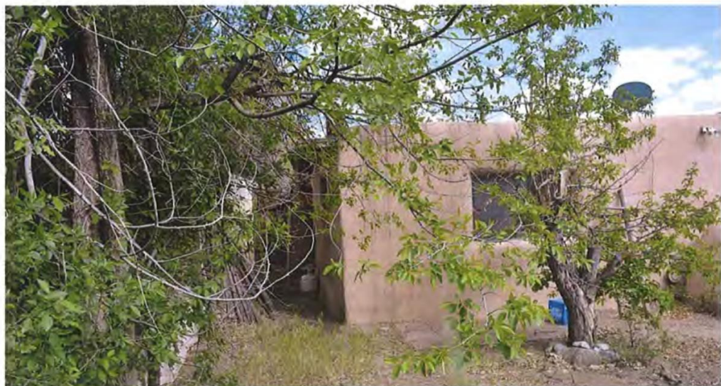
Photo 4: East and north elevations, facing southwest (top); west and north elevations, facing east (bottom).
