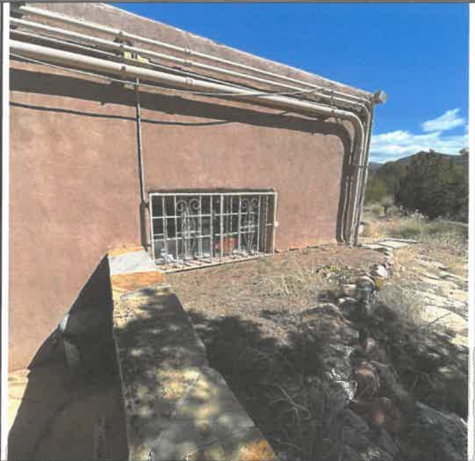
1b. This view shows some of the existing electrical conduits on wall. All exterior electrical conduits and lighting will be evaluated to see if we can remove any abandoned flood lights and conduit.
