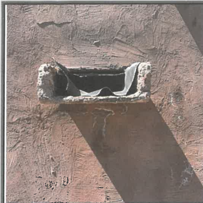
6a. This view shows the existing deteriorated concrete canals.
