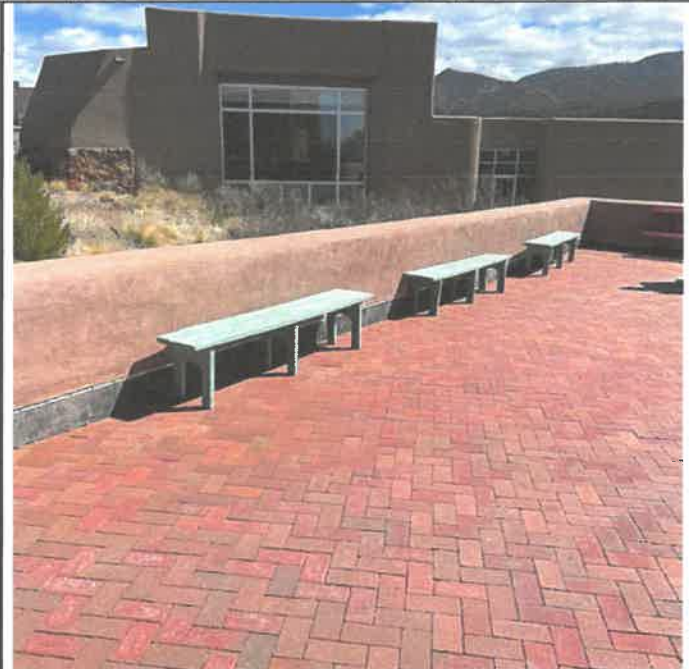
4b. 6" will be added to the top of the wall to comply with required 42" height per code. Stucco will match existing.
