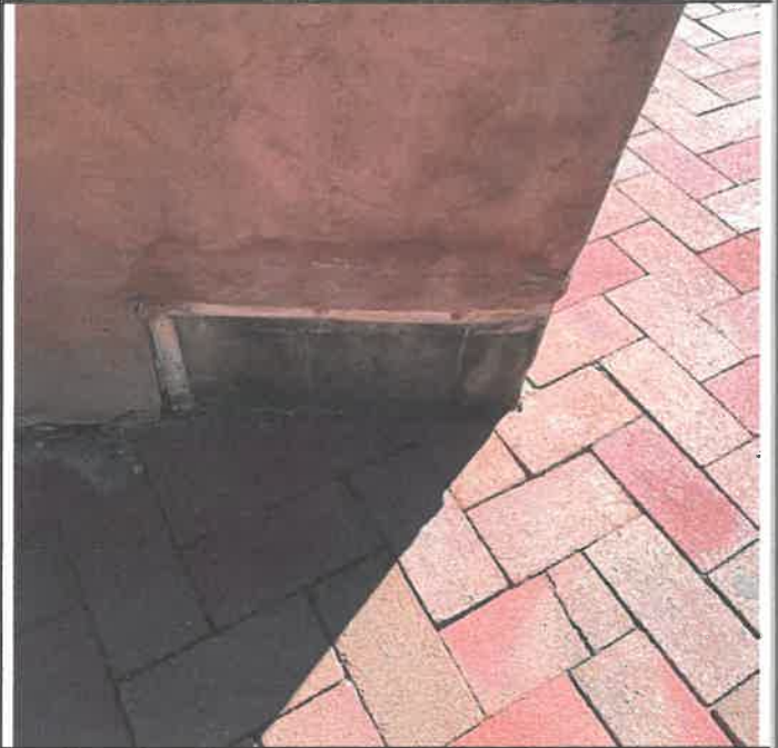
2b. This view shows a close up of the wall flashing and term bar. This will be replaced by a copper two piece counterflashing, as per original design.
