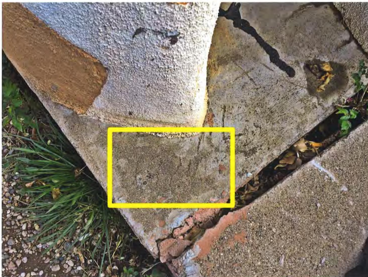
Photo 5: Scratched inscription on concrete of non-historic porch. The inscription appears to be "1994."
