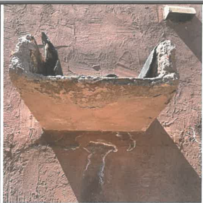
6b. Deteriorated concrete will be removed and replaced in kind. Metal canal liner will be added.
