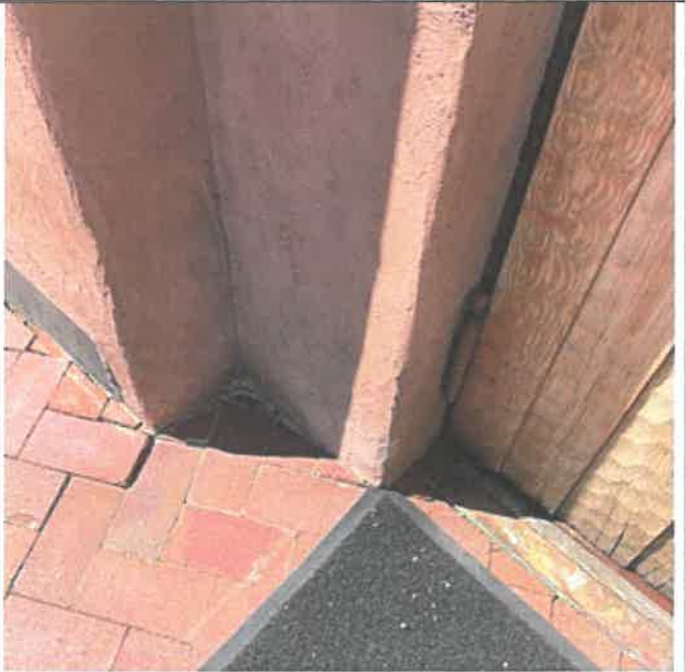
5b. Door and threshold will be replaced to match existing. Brick pavers will be sloped away from threshold to prevent ponding water. Threshold will be copper to match existing.
