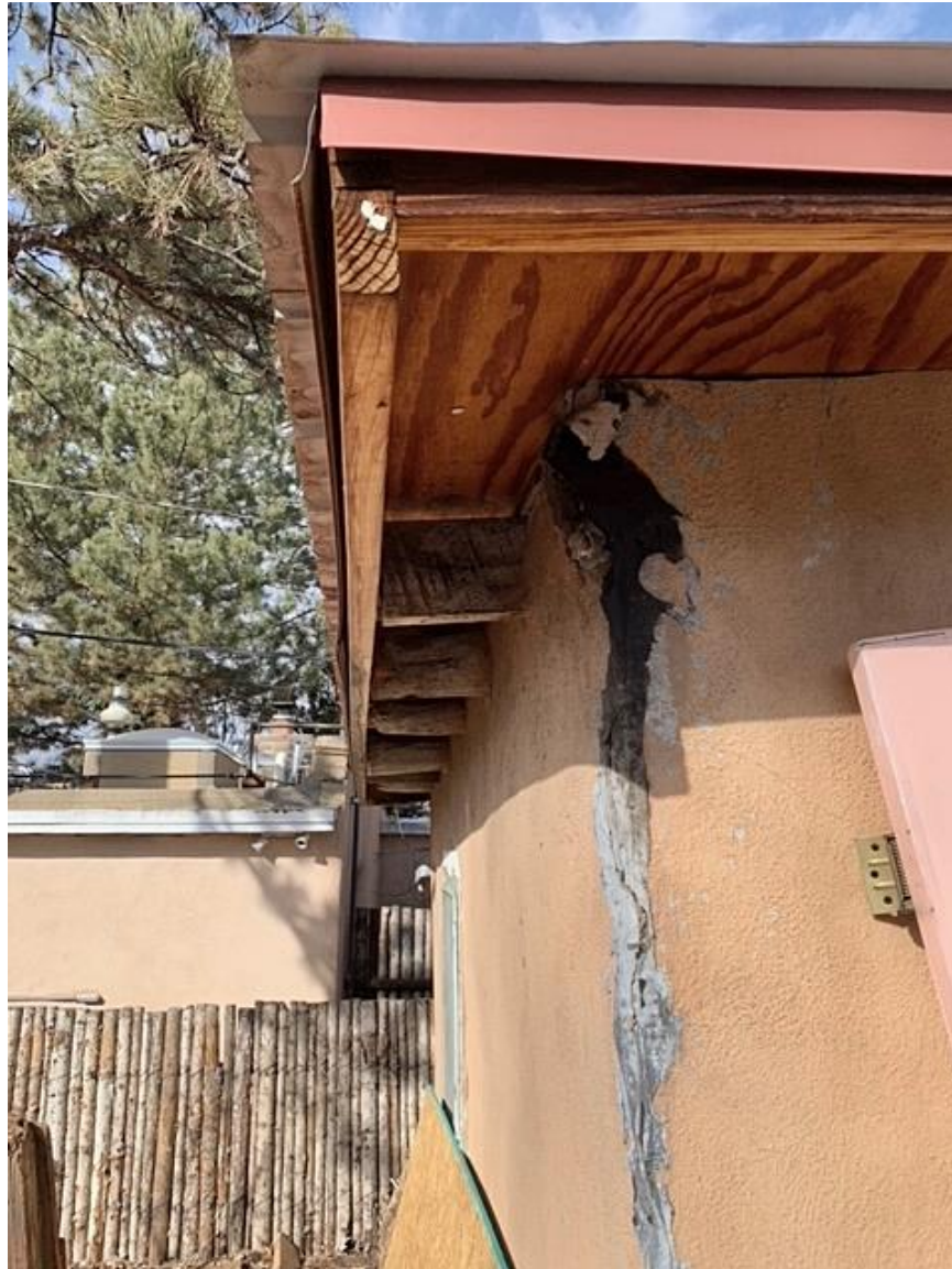
Photo 3: Southwest corner. Example of cracking and view of plywood roof decking. Camera facing up. Douglas Maahs, February 6, 2023.
