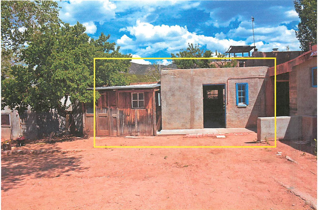
Photo 12: Building C: West elevation, facing east. Box indicates extent of non-historic CMU infill.
