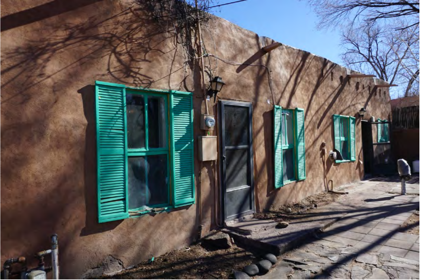
ANOTHER VIEW OF THE SOUTH FACADE WITH PROTRUDING METAL CANALES, THE EXPOSED BEAMS, AND THE FALSE SHUTTERS.
