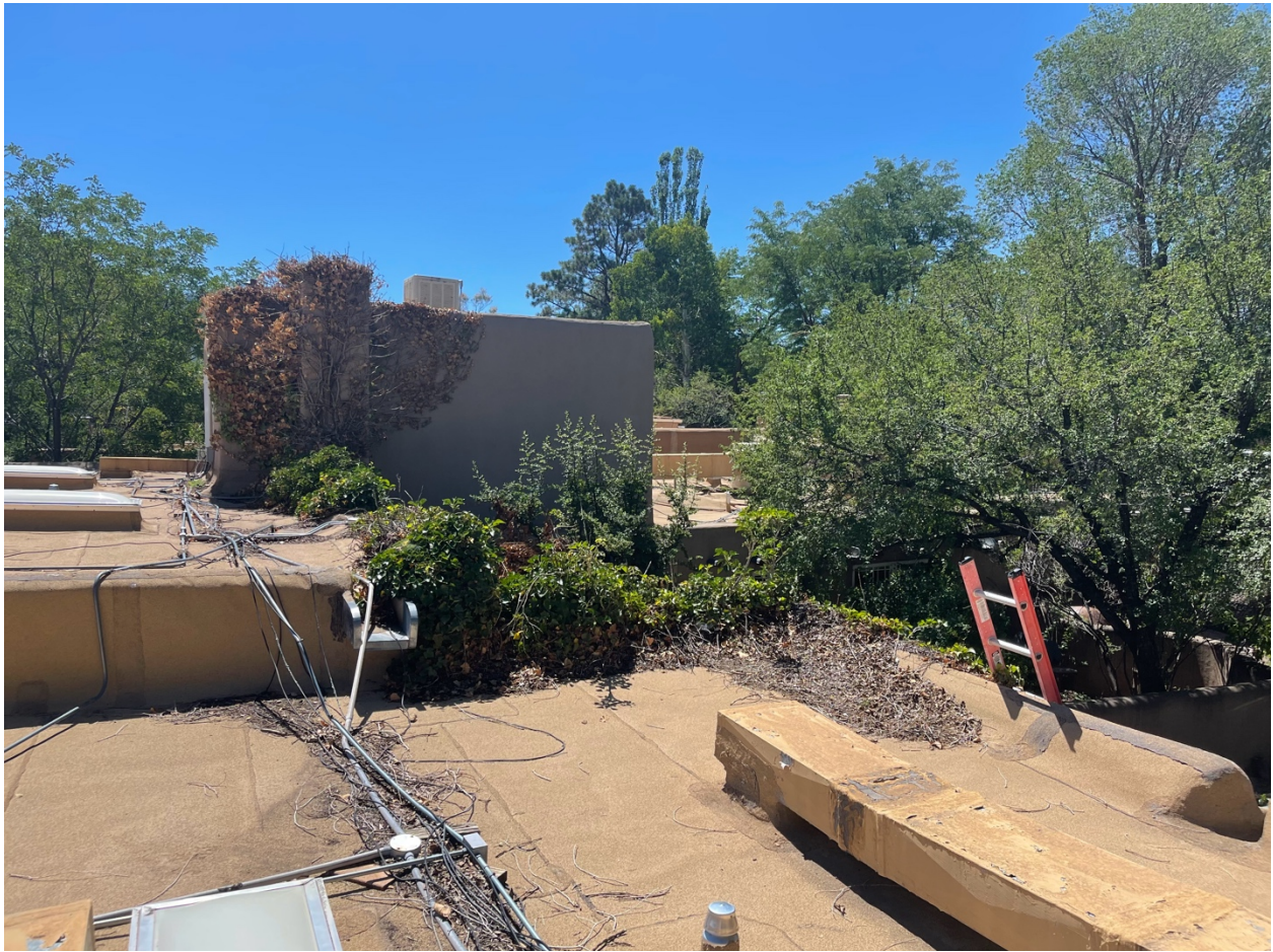
Roof top view looking east showing the roof line of the gallery, former studio, and the second floor.
