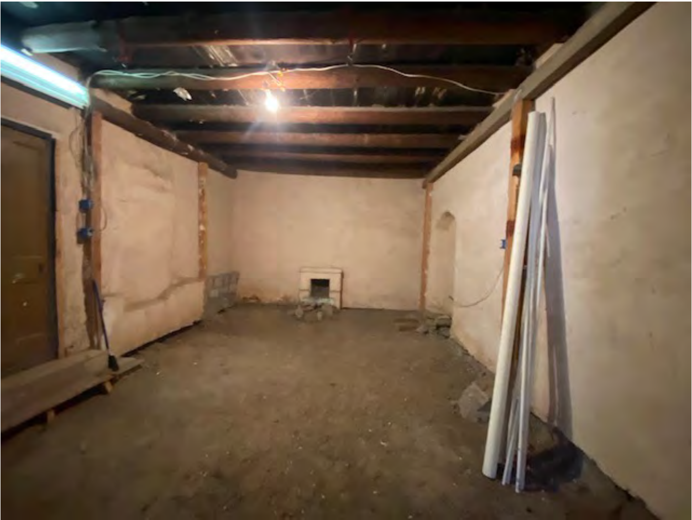
Interior of Unheated Storage Room on North with Fireplace without a flue, arched niche, CMU and Concrete pads supporting new wood frame at vigas at both bearing points. See blocked window on the left.
