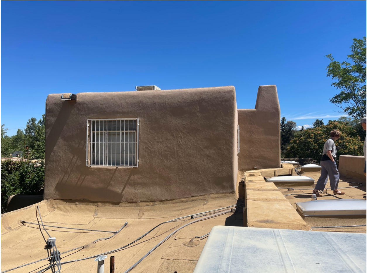
Roof top at second floor. Notice attached chimney of kiva below. Steel casement windows at second floor.
