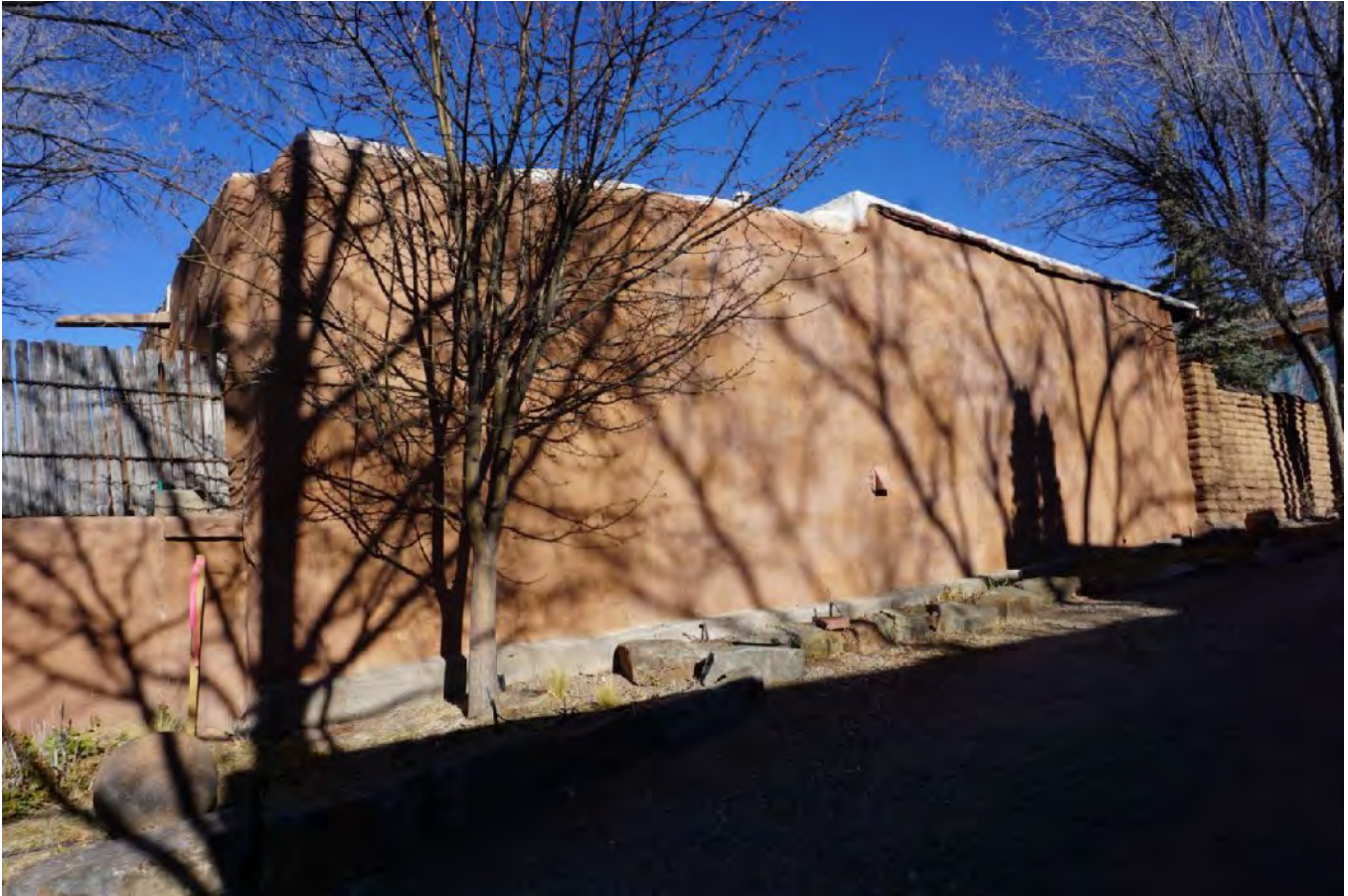
EAST FACADE WITH NO OPENINGS, CONCRETE CURB ADDED, FIBERGLASS FROM ROOFING VISIBLE ON PARAPET. PRIOR TO 1966 BUILDINGS ALONG THIS LINE
