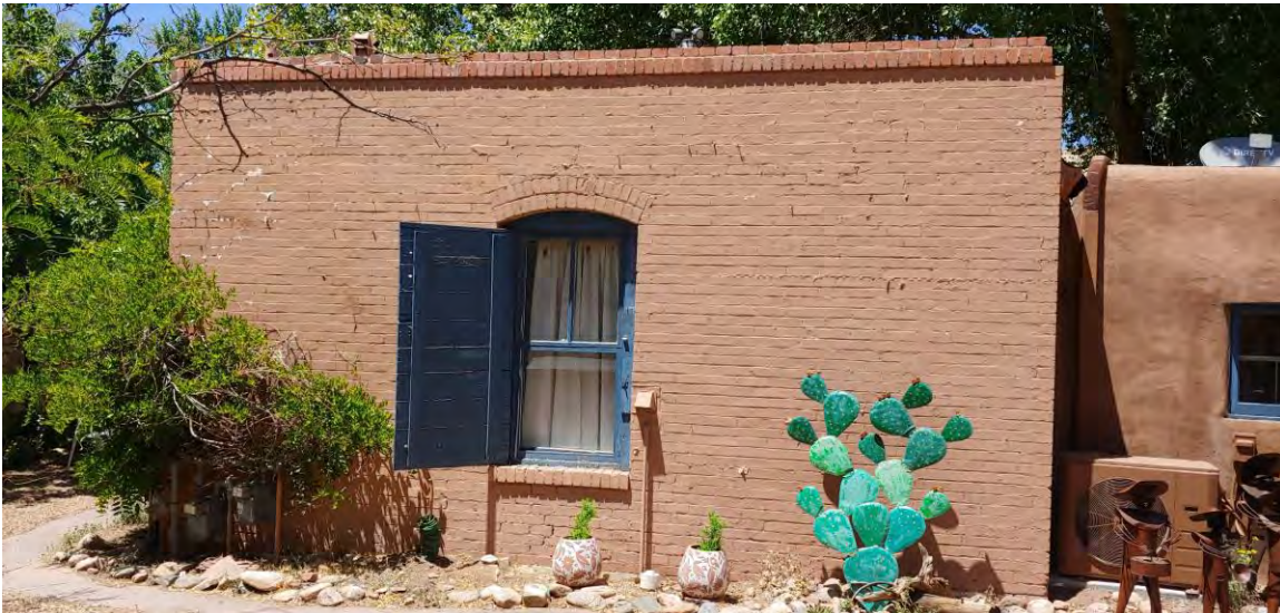
Photo 3: View of Cider Press, south elevation, original garage portion. Camera facing north.
