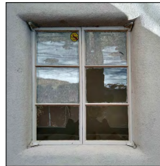
STEEL WINDOW NO LINTEL
