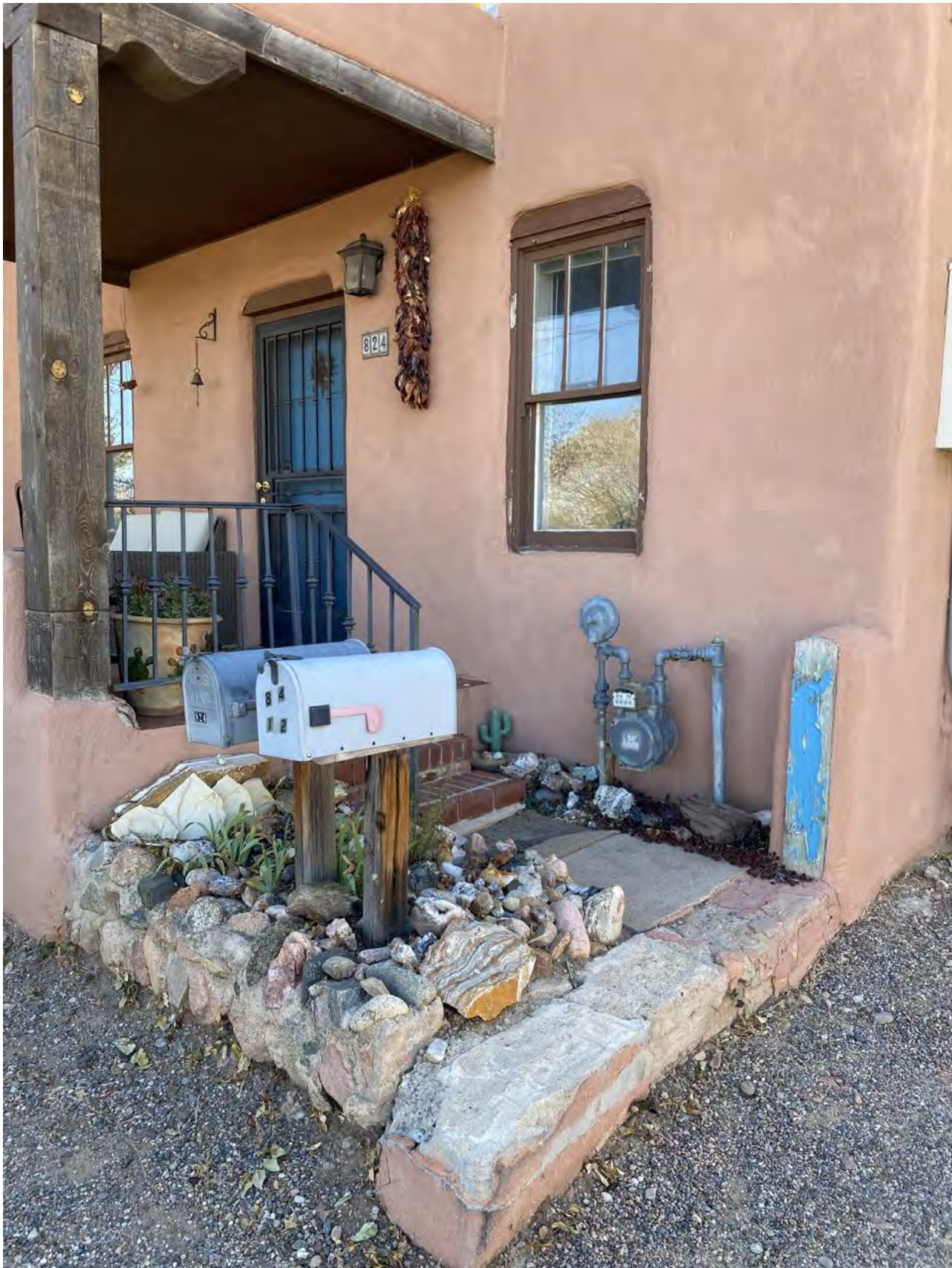
PROPOSED NEW CONCRETE STEPS WIDTH OF PORTAL - REMOVE HODGE-PODGE ROCK PLANTER / MAILBOXES
