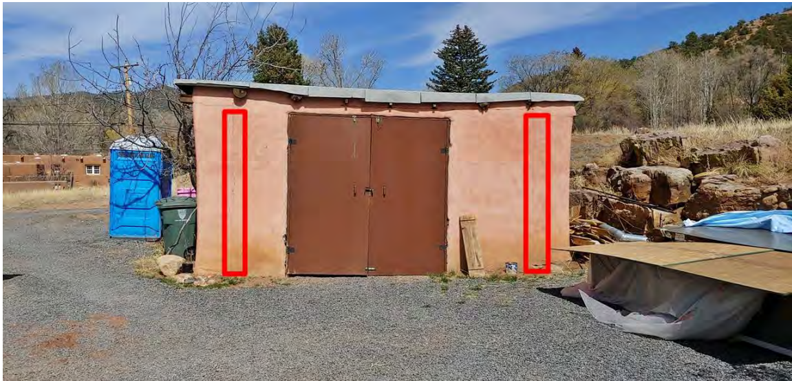
Photo 7: West elevation. Vertical cracking highlighted. Camera facing east.
