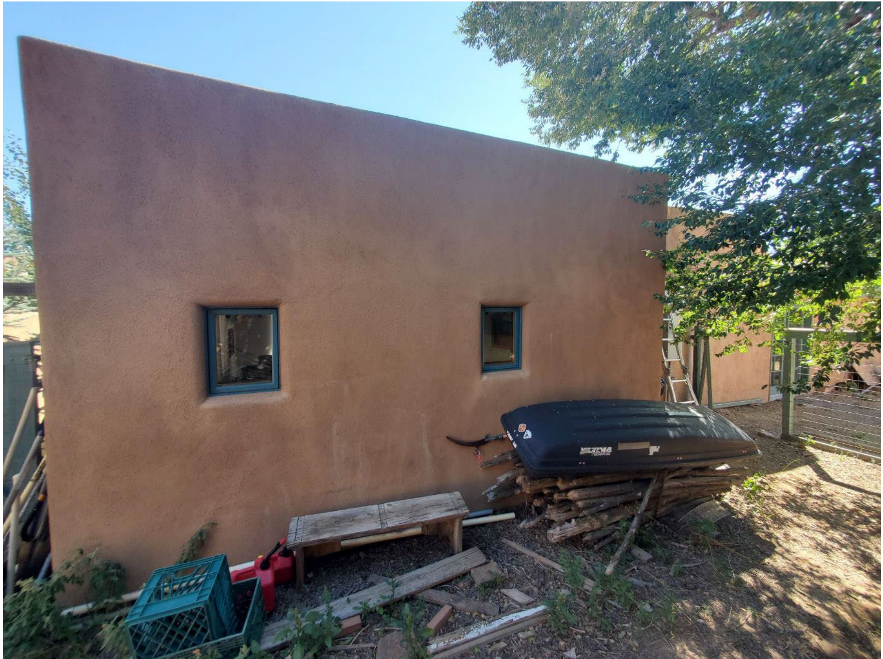
1224 ½ Cerro Gordo: North Elevation 1 (distortion from lens because can't get very far away from house)
