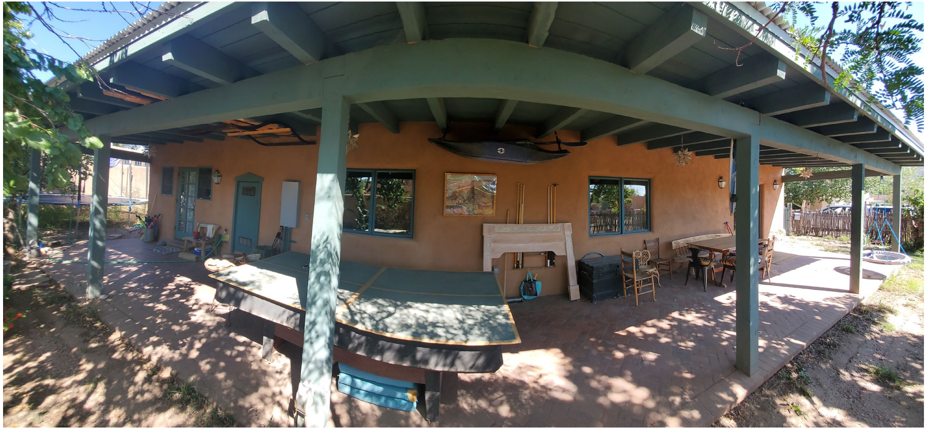
1224 ½ Cerro Gordo: West Elevation (panorama, straight wall and portal “bent” by camera)
