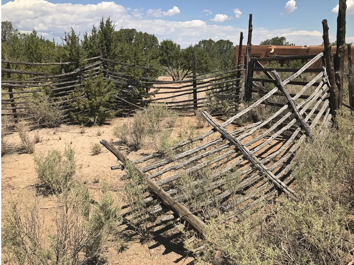
Photo 16: Small Corral-Round Pen, damaged panels. Camera facing north.
