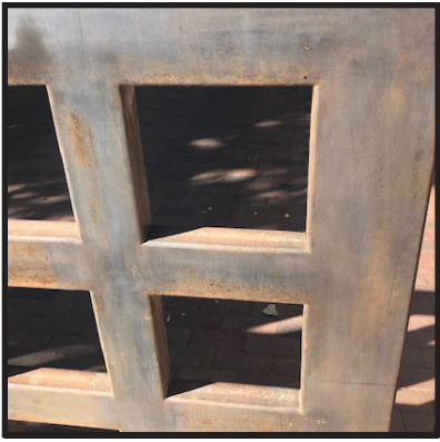
RUSTED (OXIDIZED) STEEL FRAME
