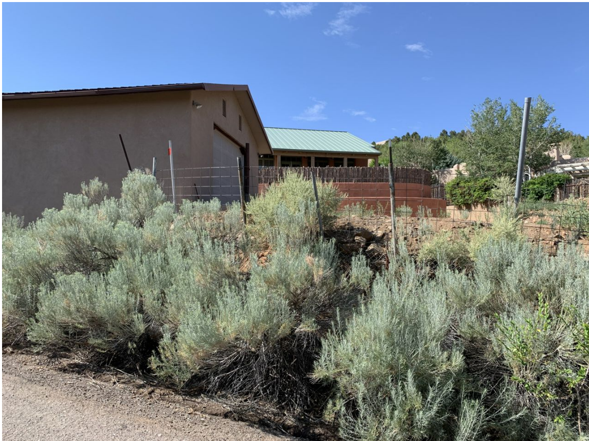
EXISTING WIRE FENCE SUPPORTING DIRT
