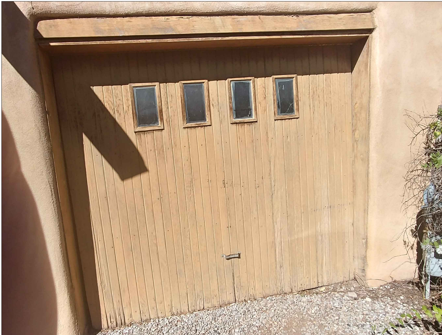
Garage door condition
