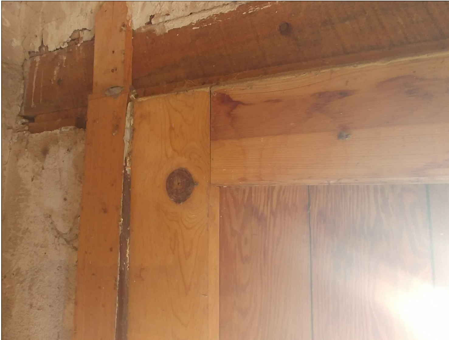
Garage door condition
