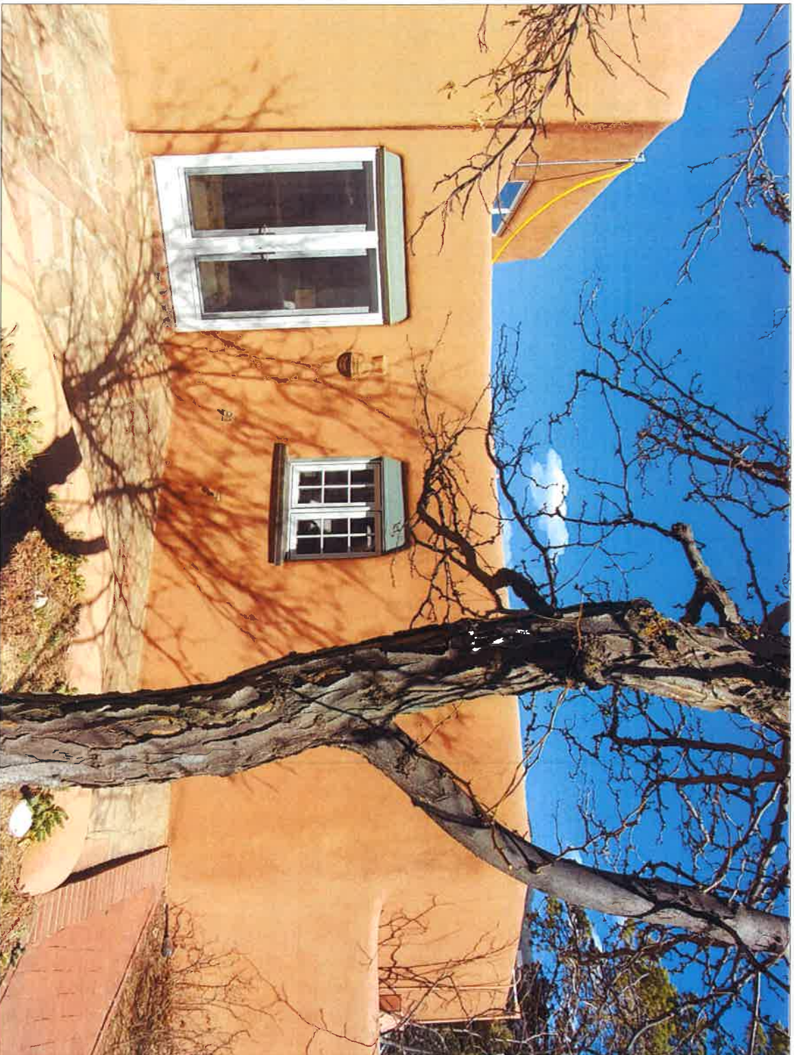
Area of proposed formal entry, portal, steps and flagstone walkway looking east
