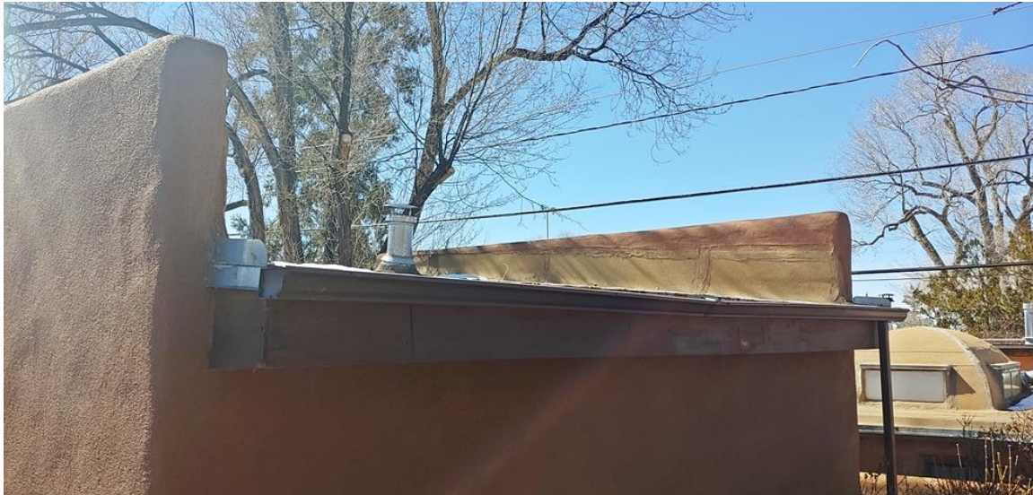
Photo 15: Garage, roof. Note extended parapets at east and west elevations. Camera facing southwest.
