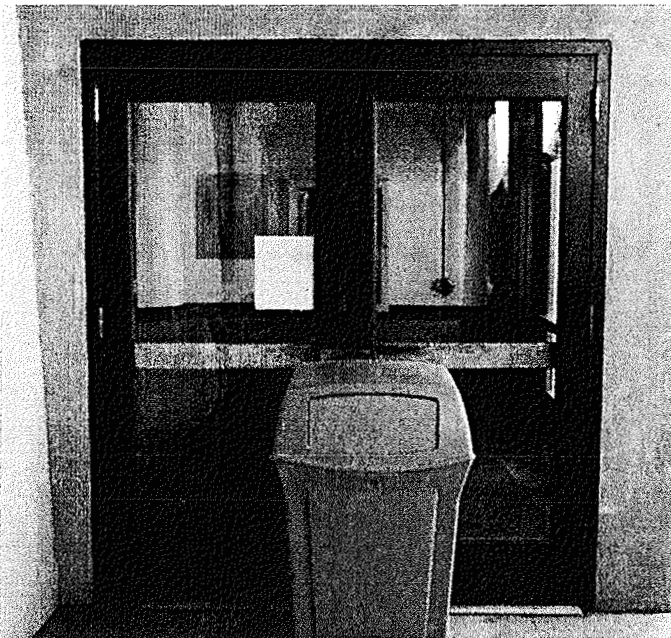
D3 (blocked main entry vestibule)
