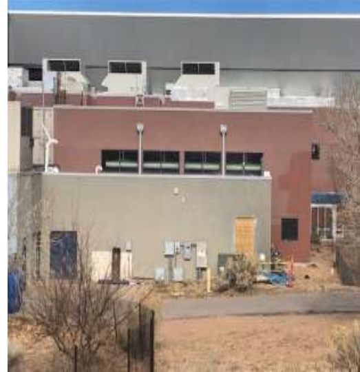
GCCC New Roof Top Units
