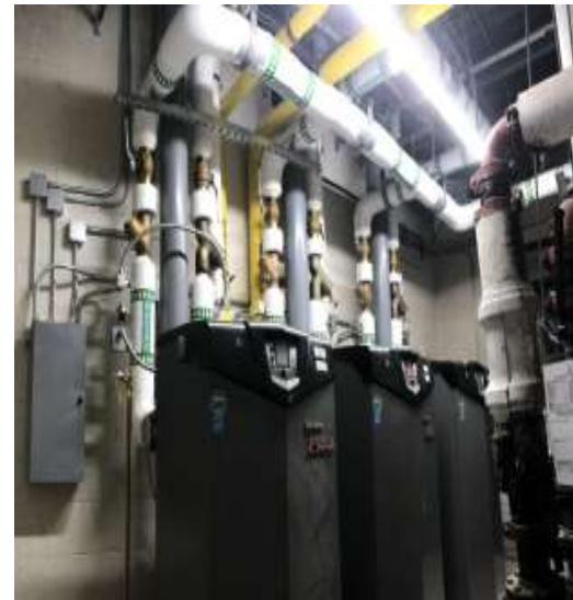
GCCC New Boilers
