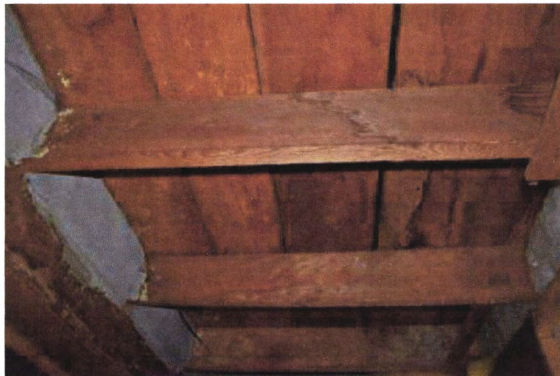
Photo 8: Garage - interior. Altered west section (top); original east section (bottom). Camera facing up.
