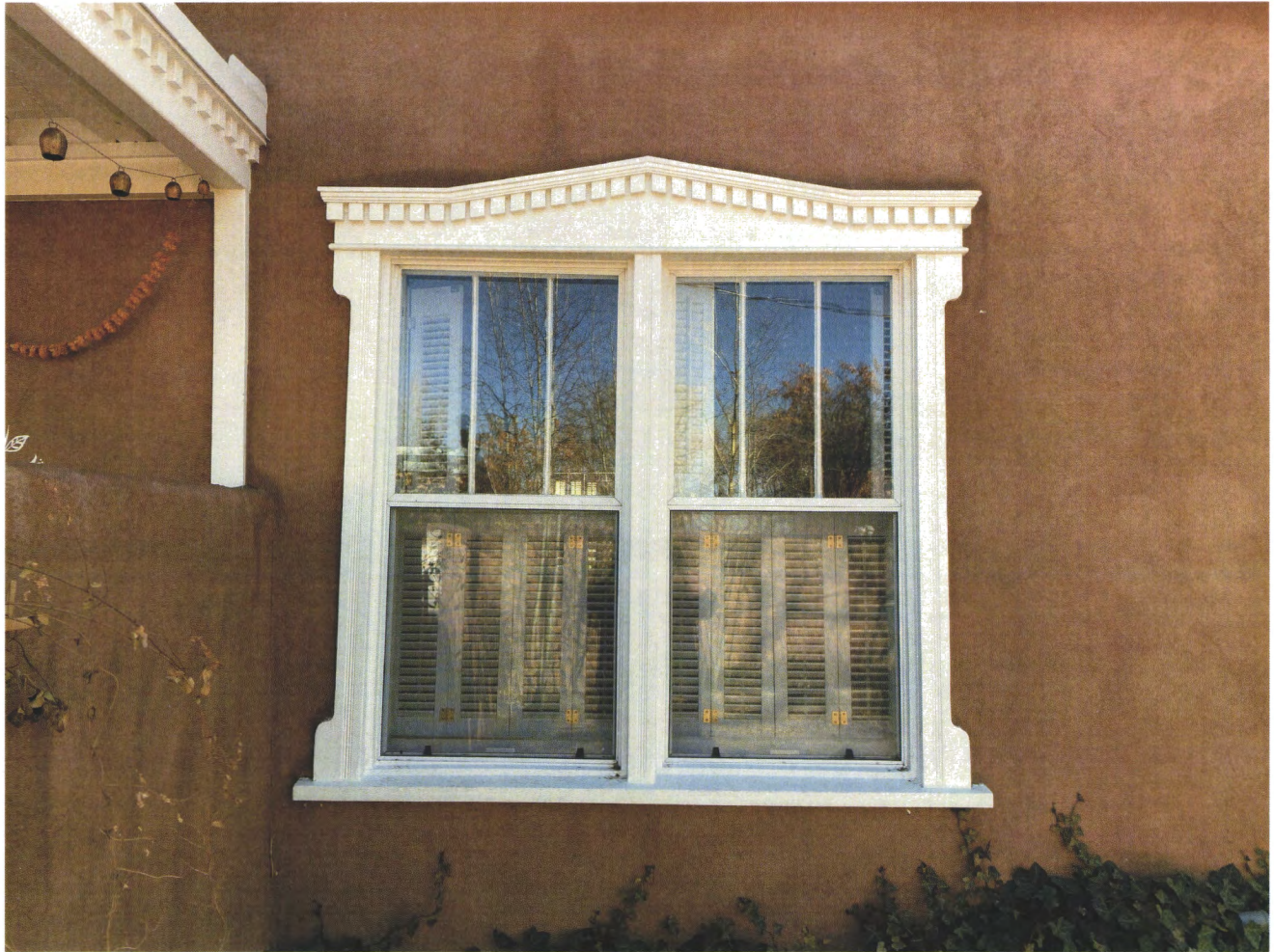
EXISTING WINDOW @ EXISTING RESIDENCE – New window along street front to match existing Territorial style; painted wood.
