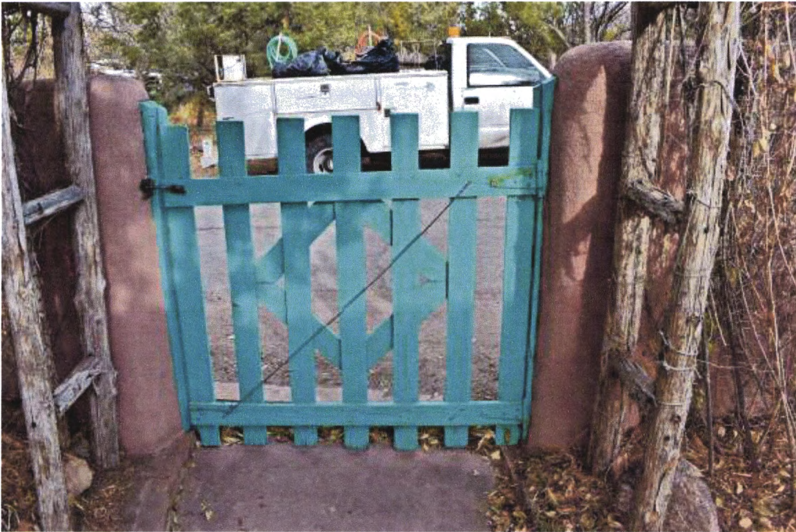
Photo 3: Street Wall, entry gate. Note gate has seven vertical slats. Camera facing east.
