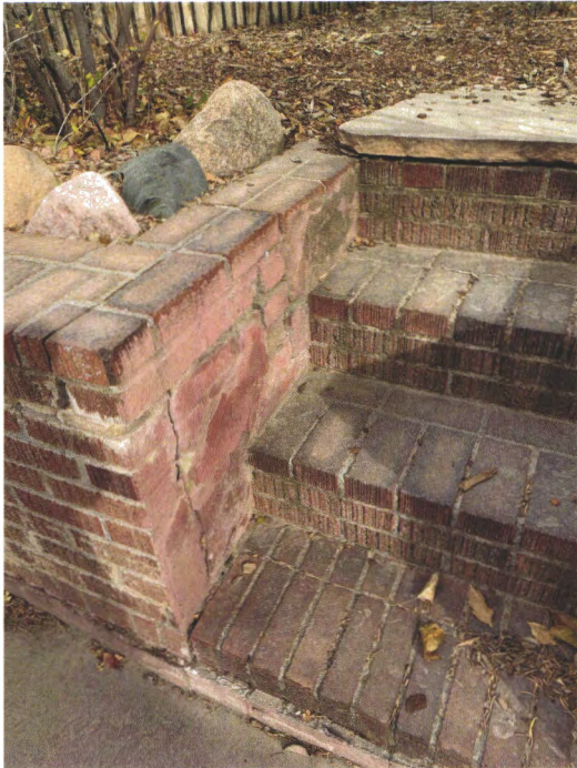
Old Stucco at Driveway Brick
