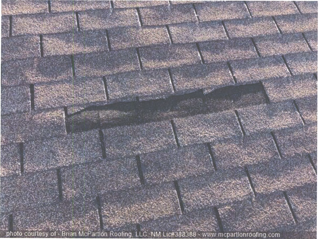
Detail of roof damage
