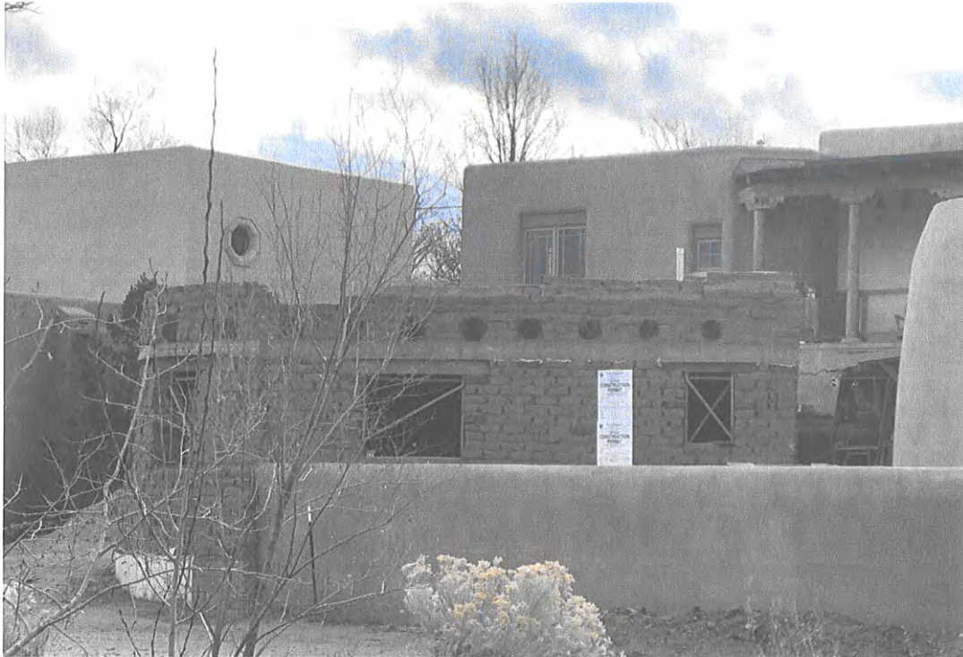
5. North side of adobe studio and yard wall – looking south from River Park
