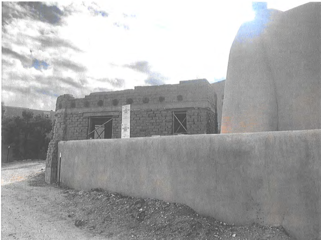
6. North side of adobe studio and yard wall – looking southeast from lane
