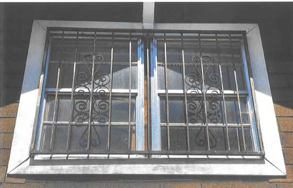
East Façade: 2nd story windows, aluminum single hung, proposed to replace 225 E Marcy St
