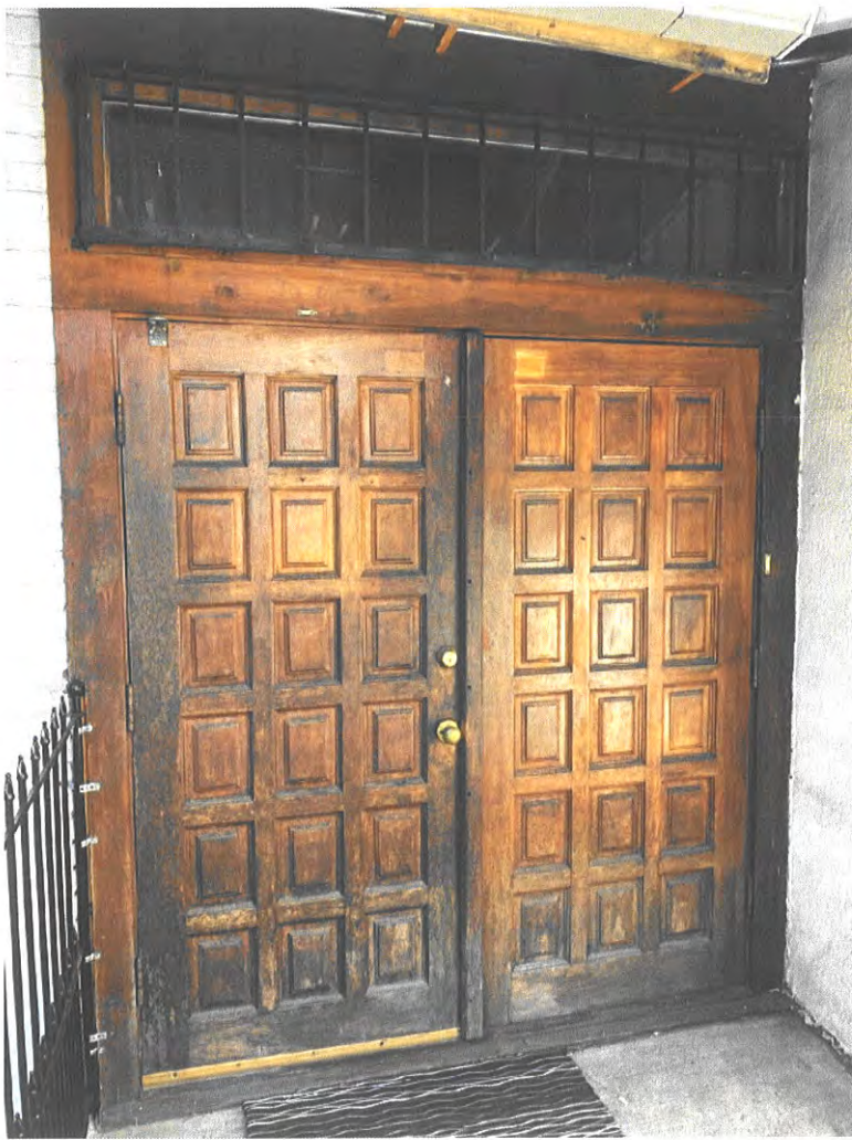
North Façade: Double doors replaced original single door in approx 1991, , proposed to replace
