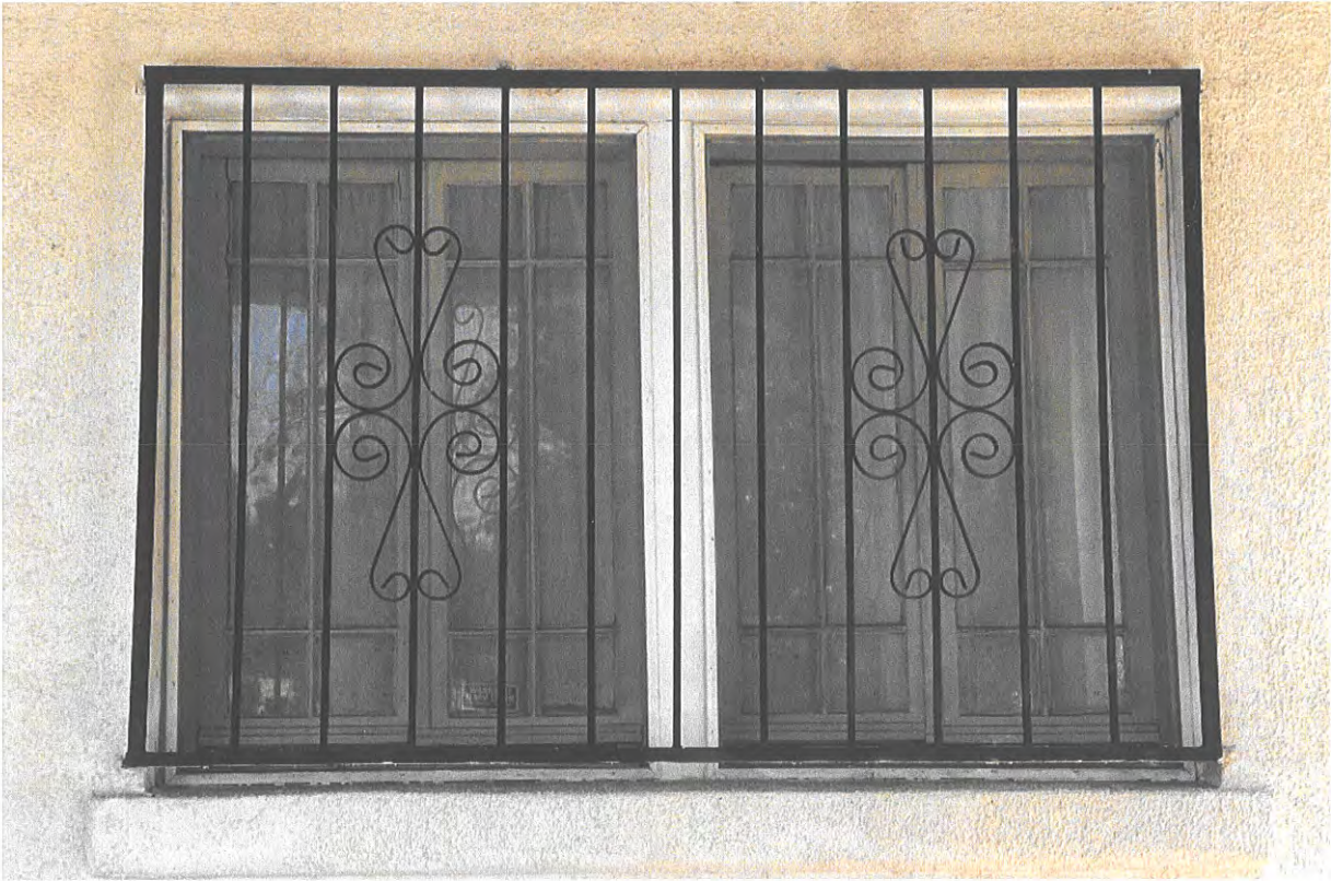
South Façade: Windows E of doors, example of metal grates proposed to be removed
