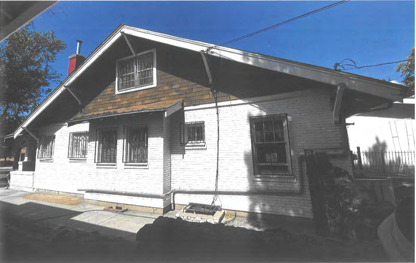
225 E Marcy St East Façade viewed from NE, Primary facade, note asphalt shingle siding covering historic cedar shake
