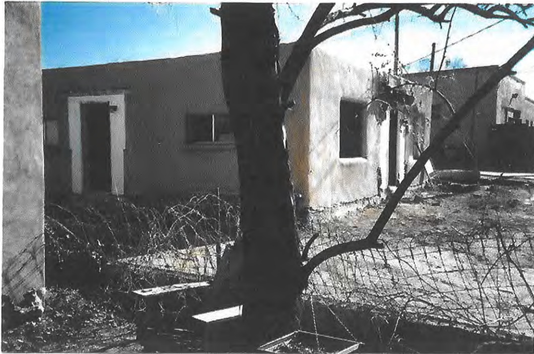
Figure 10: 2002 construction photographs. West and south elevations. Note existence of west elevation door and removal of front portal. Courtesy property owner.
