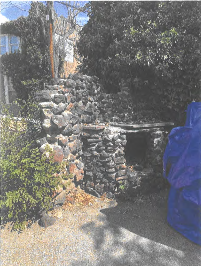
Lava rock wall / fireplace at NE corner of lot in disrepair proposed to be removed for ADA parking 225 E Marcy St
