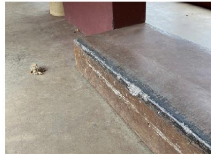
Damaged concrete bench at Marion-Tipton portal walkway.
