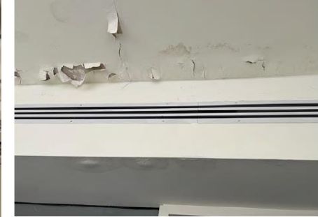
Evidence of roof leak at ceiling, Tishman 111A - Library Nook
