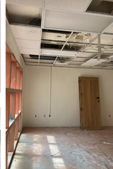
Damage to ceiling, floor, and windows, Tishman 132
