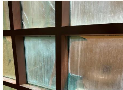
Window damage in Tishman Seminar Room 132.
