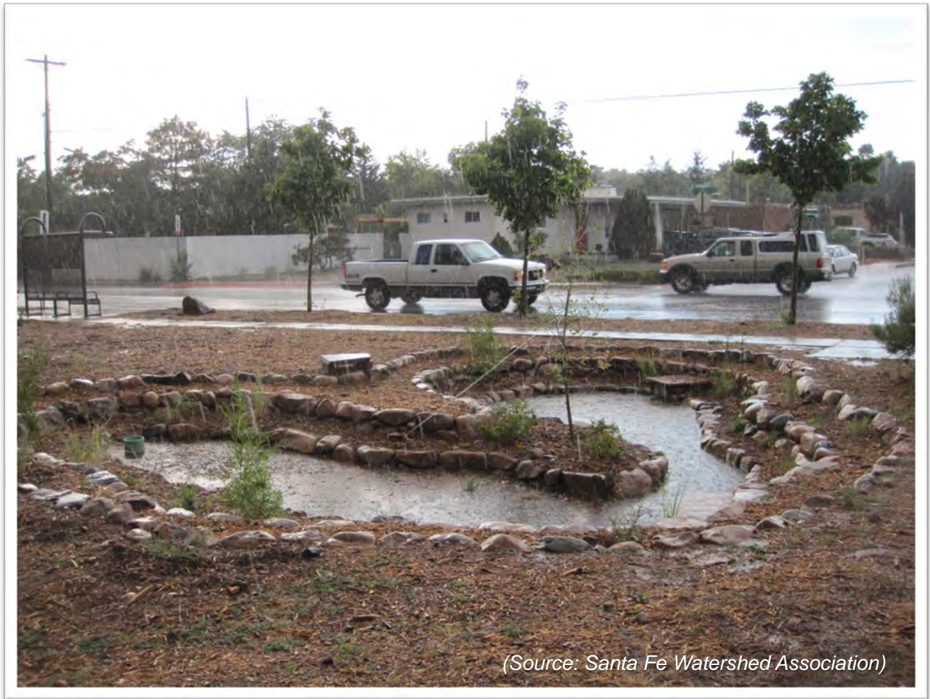
Figure 64: Bioretention Basin, also known as a Rain Garden, along West Alameda in Santa Fe
