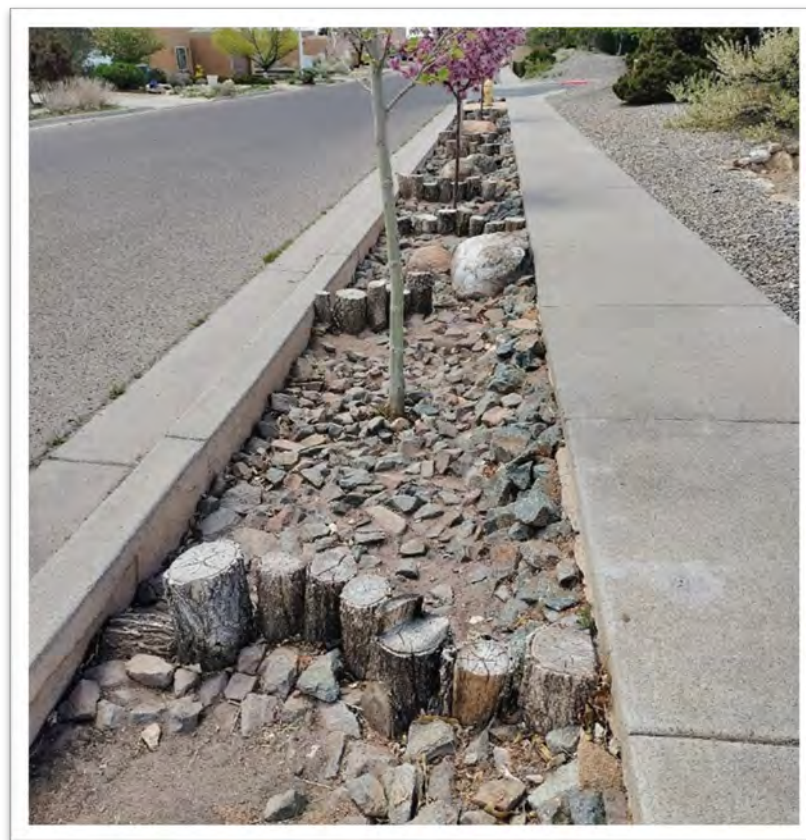
Figure 73: Check Dams Made from Wood
