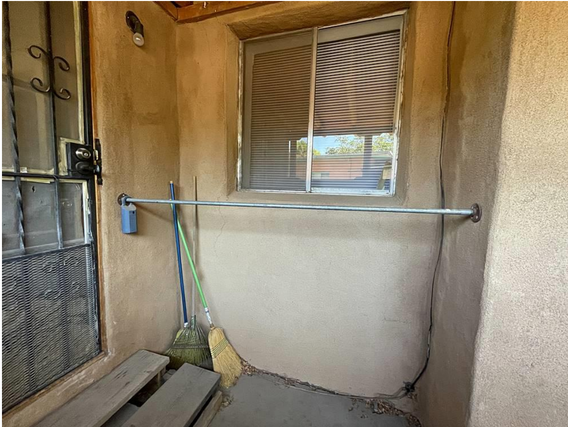
Photo 8: West elevation. Older home and entry to laundry room addition. Camera facing northeast.
