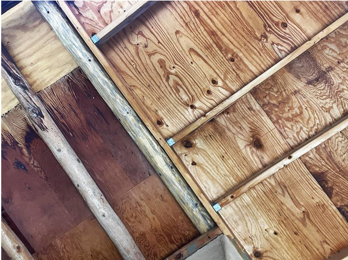
Figure 5: Joining of two non-historic porches at southwest corner of south (front) elevation. Camera facing up.
