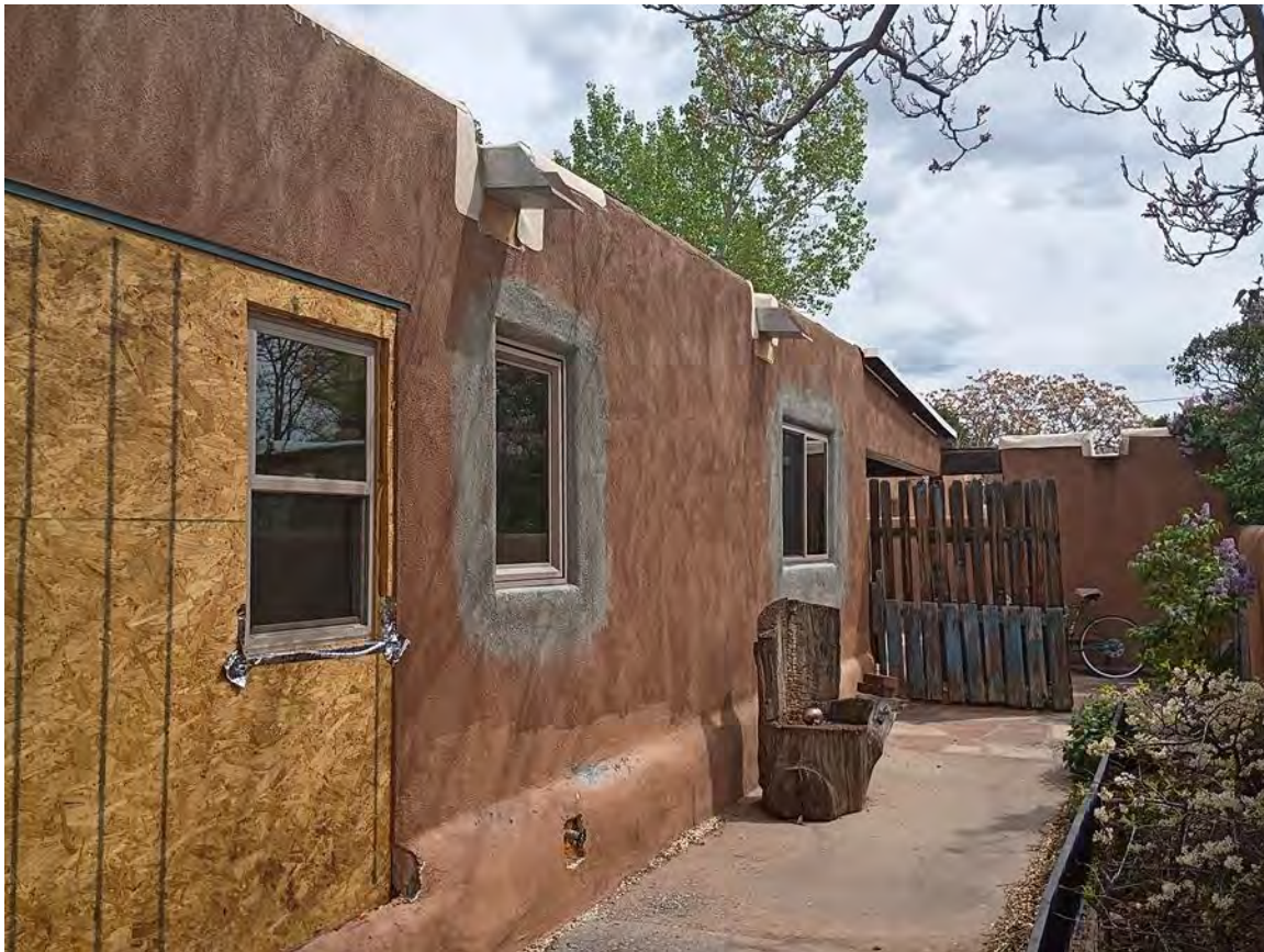
Photo 11: West elevation. Note introduction of OSB sheathing and replaced windows Camera facing southeast.
