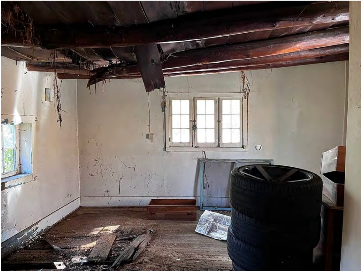
Photo 28: Bedroom. Ceiling and floor damage. Camera facing southwest.
