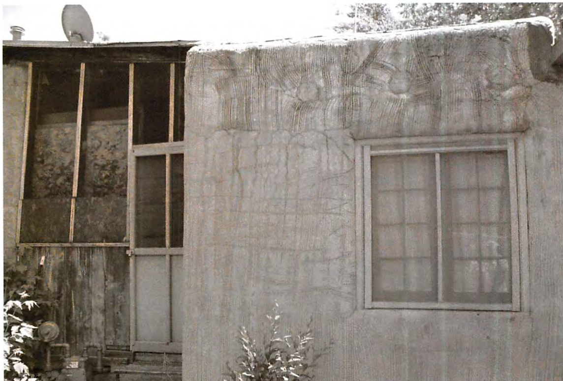
7. View South of North elevation room addition and vernacular porch (ArcCom June 5, 2007).
