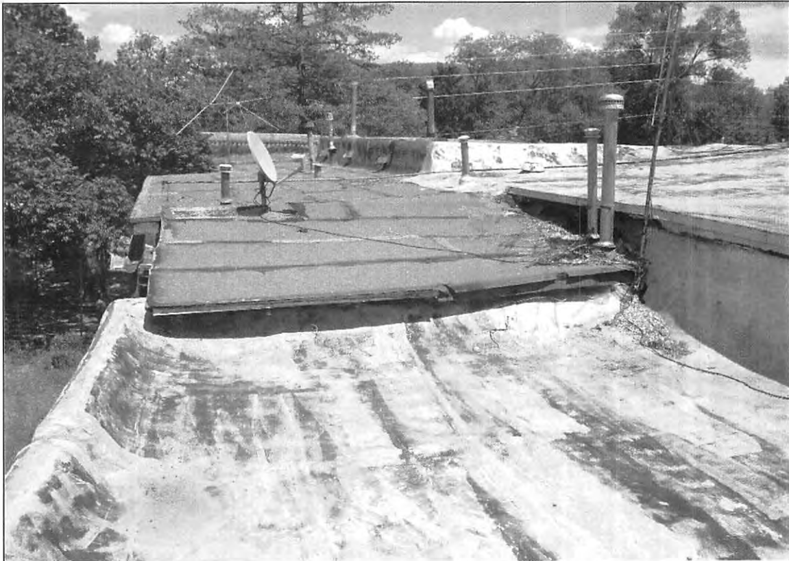
8. View East from Northwest corner. Raised parapet in distant right is believed to represent original (1890s) footprint (ArcCom June 5, 2007).
