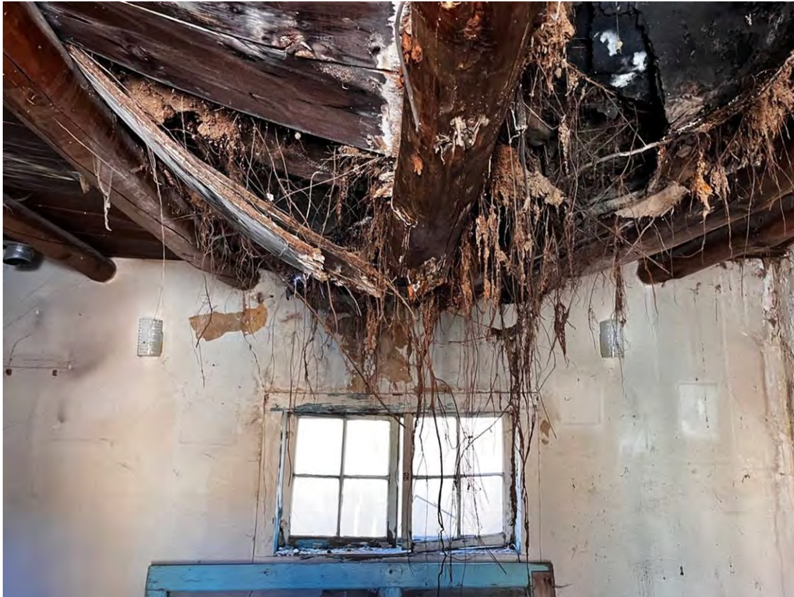
Photo 28: Living room. Roof and ceiling damage. Camera facing up.
