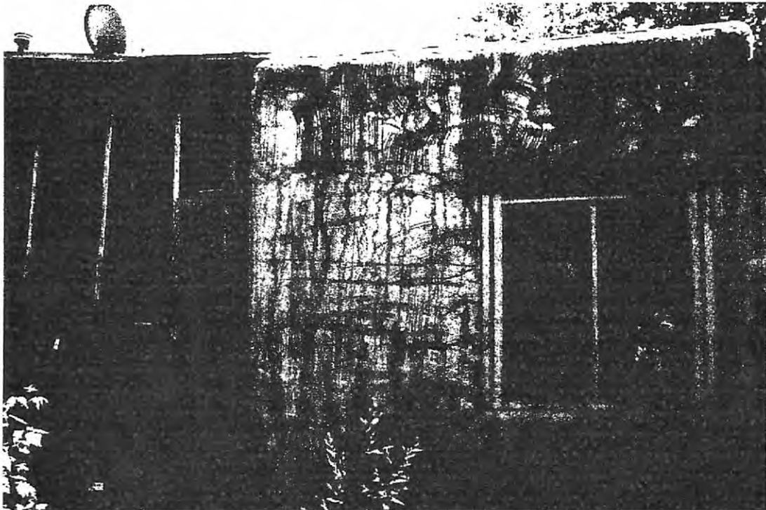
7. View South of North elevation room addition and vernacular porch (ArcCom June 5, 2007).
