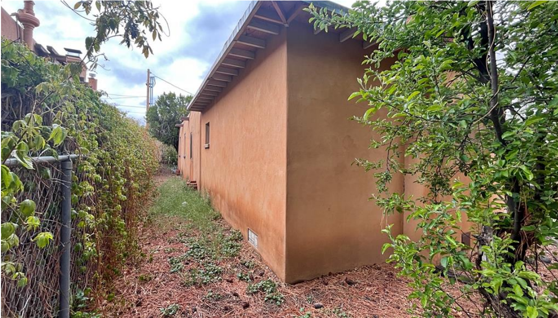
Photo 20: East elevation oblique from north end. Addition in foreground. Camera facing southwest.
