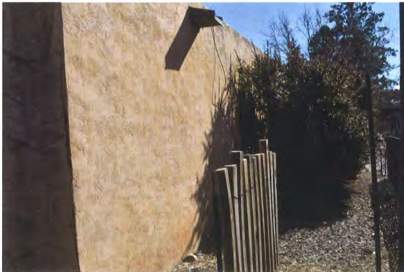
Photo 2: Street and west elevations (top), facing northeast; west elevation, facing south (Sharon Joyce, February 23, 2018).
