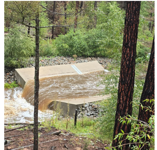
> Santa Fe River flows over flume above McClure during record high flows in September.
