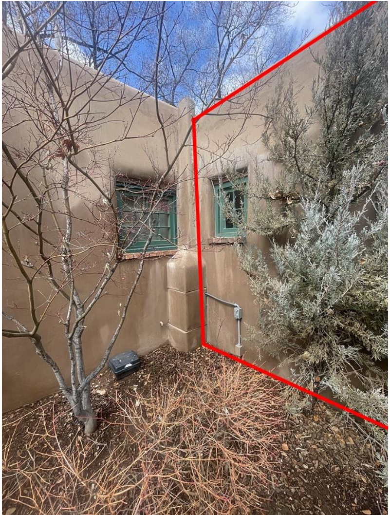
Photo 6: East elevation, c.1994 portal entry addition outlined in red. Camera facing northeast.
