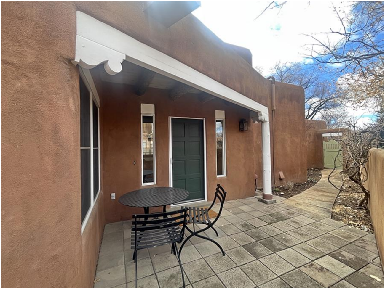
Figure 2: North (front) elevation of subject house, camera facing southeast. February 14, 2026. Giulia Caporuscio.
