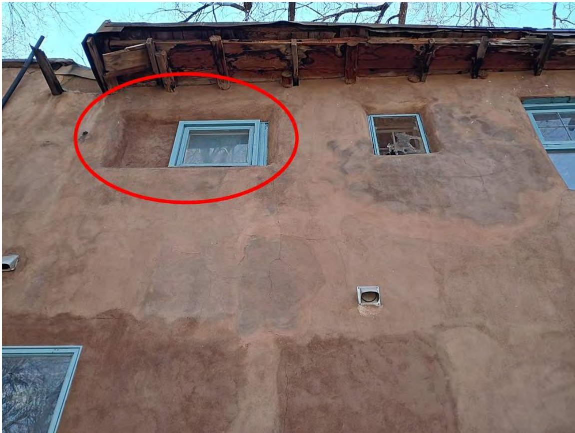
Photo 18: North elevation, window opening alteration. Camera facing up.
