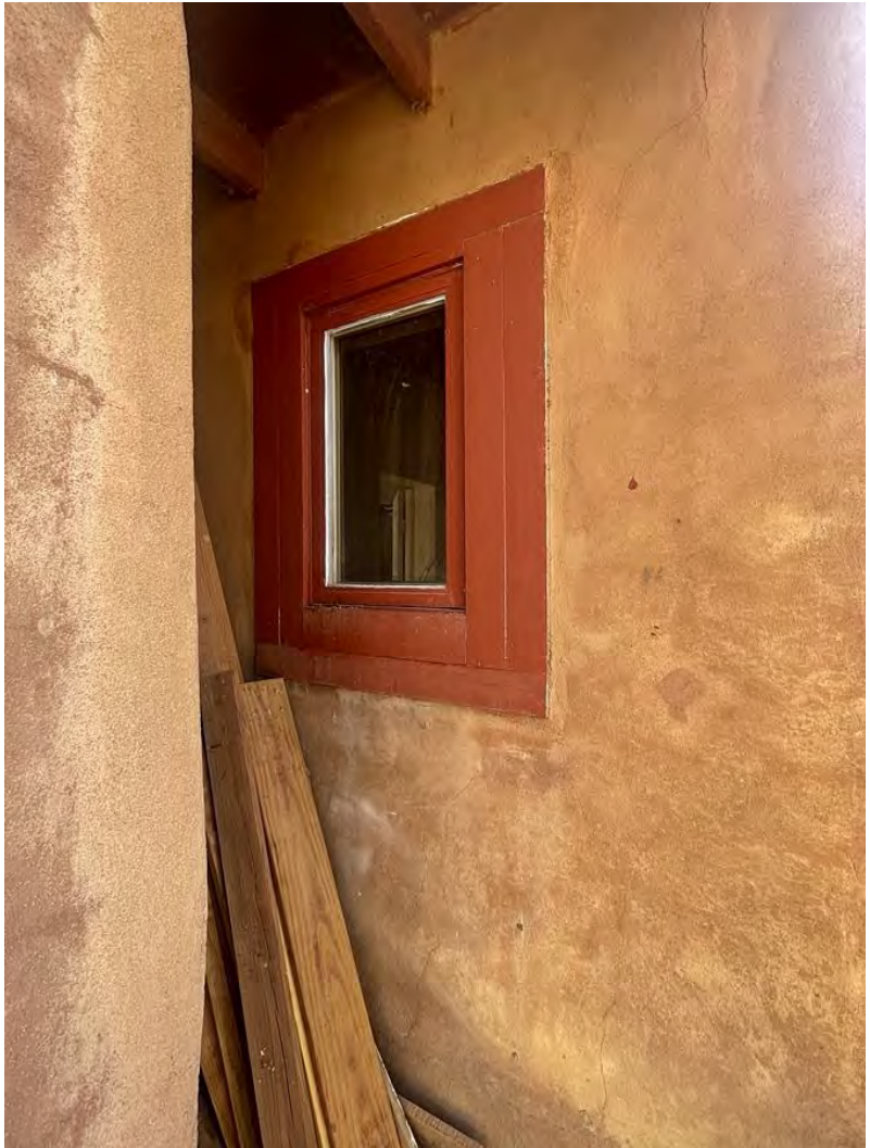
Photo 3: West elevation. Gap between non-historic addition and probable infilled porch. Camera facing southeast.
