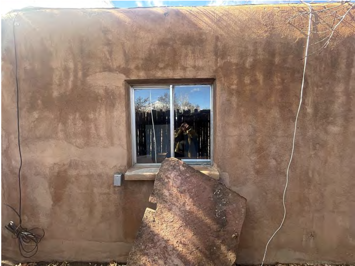
Photo 9: East elevation. Window at what may be pre-1969 addition. Camera facing west.
