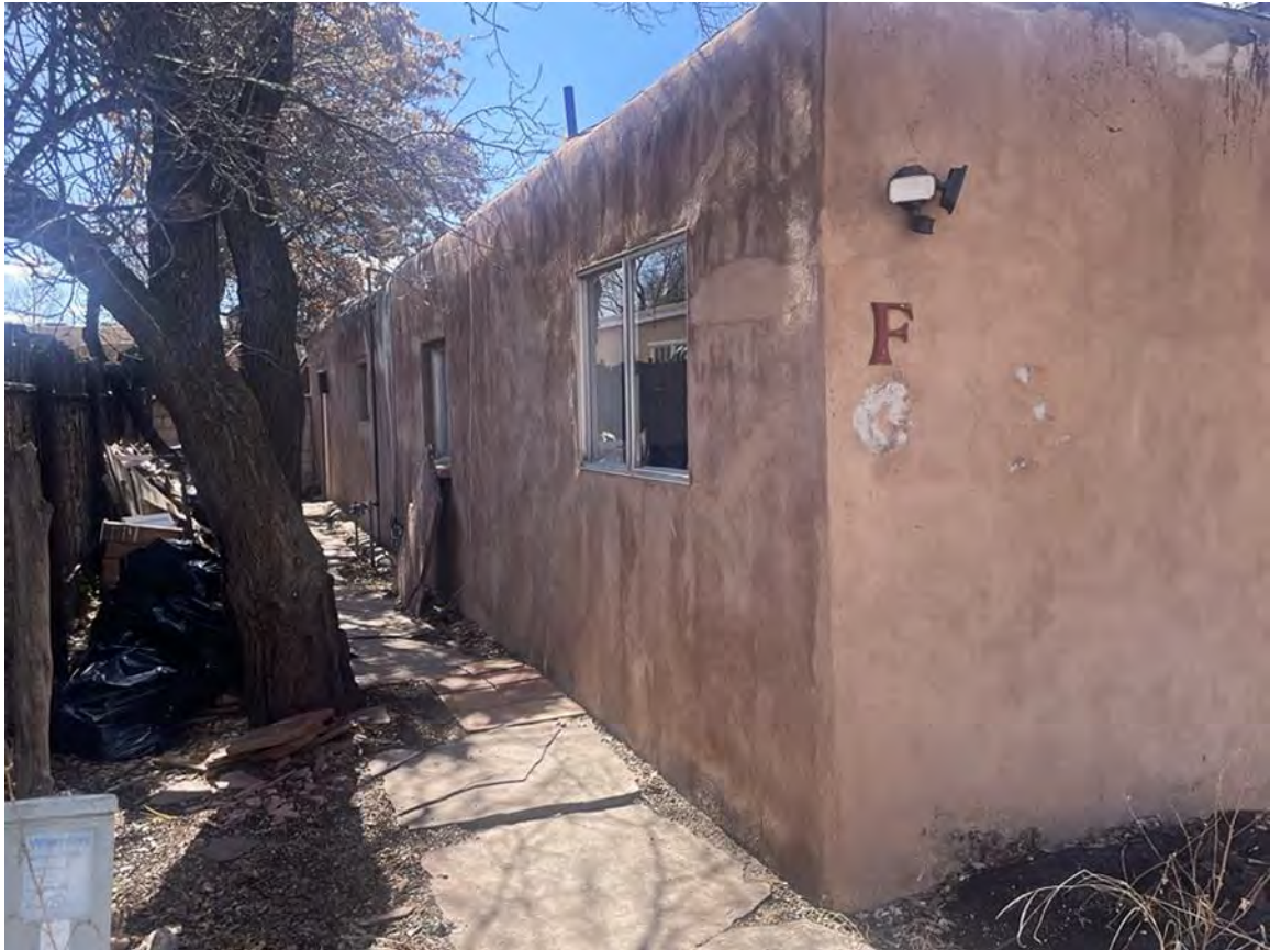
Photo 10: East elevation, north end. Window at foreground dates to the 1975-1978 addition. Camera facing southwest.
