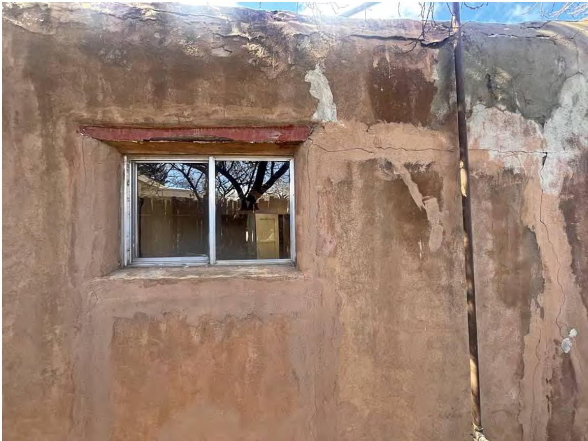
Photo 8: East elevation. Window at what may be the original core of the building. Camera facing west.
