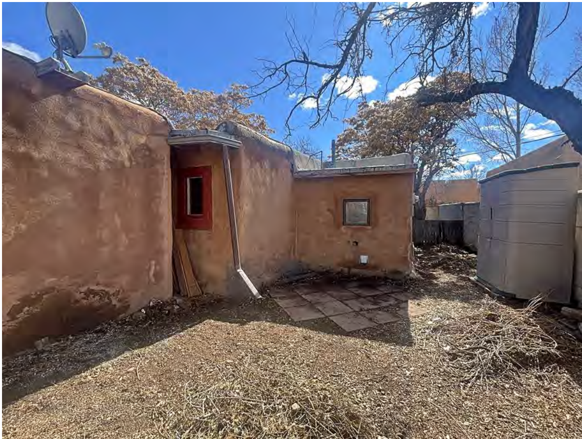
Photo 4: West elevation. Volume to the right may an infilled entry porch. Camera facing south.
