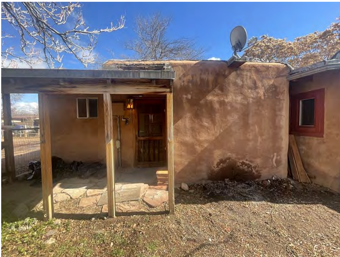
Photo 2: West elevation. Non-historic addition. Camera facing east. Note probable infilled window.
