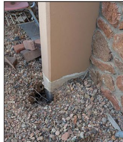
4) Exposed Building Foundation
