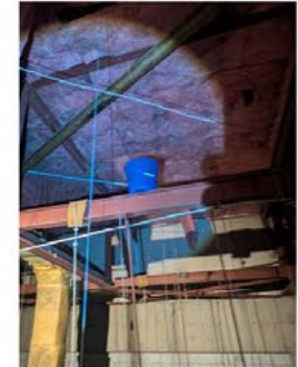
2) Leaking Roof Drain
