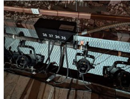
1) Stage Lighting in Attic Level
