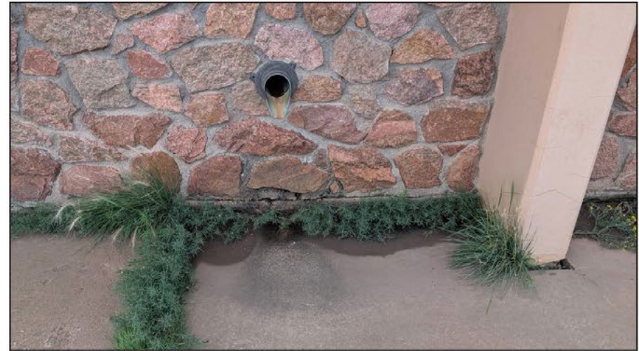
1) Roof Water Infiltration into Building Foundation
