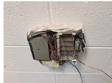
3) Telephone Equipment, Office 147
