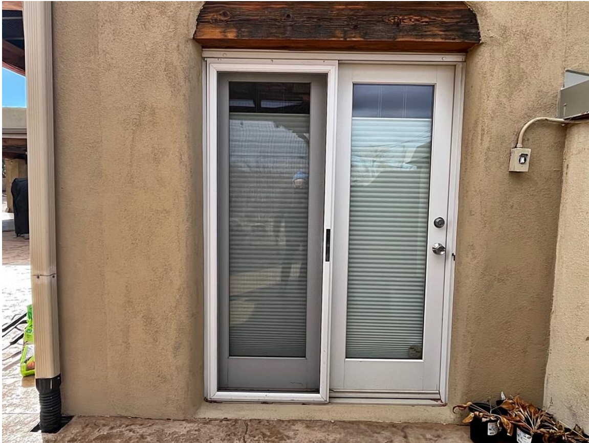
Photo 16: North elevation. Non-historic opening at primary bedroom. Camera facing southwest.
