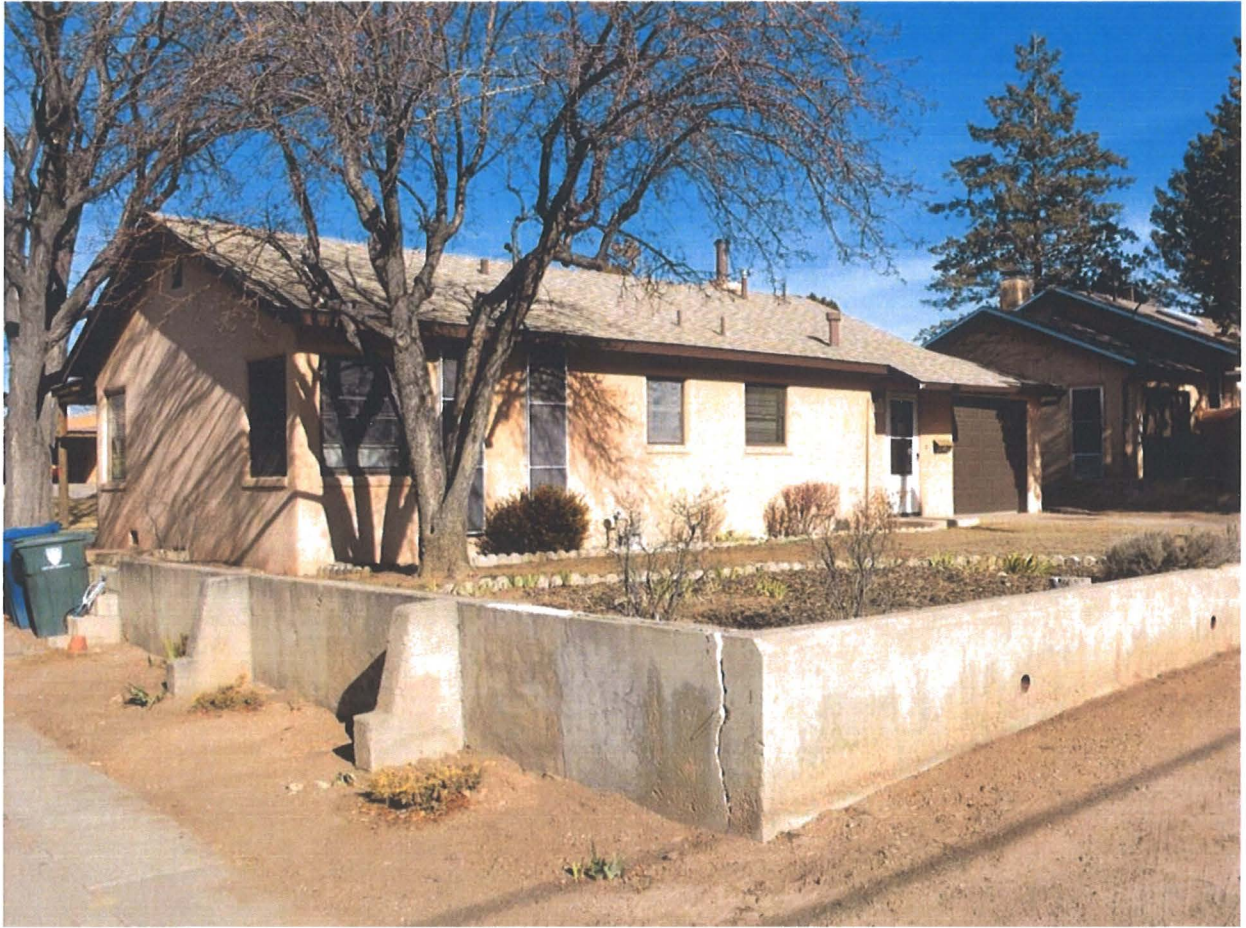
Figure 3: c.1950 concrete retaining in front of 107 Camino Matias. January 18, 2018.
