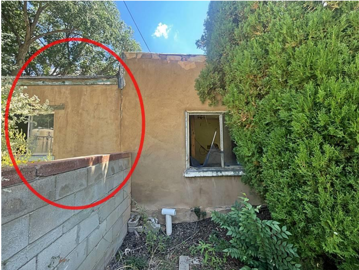
Photo 4: West elevation. Older section. Enclosed porch or patio area circled. Camera facing east.
